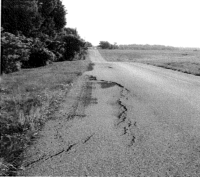
Looking east on Weichman Rd. The pavement is cracking and there is wheel rutting.
