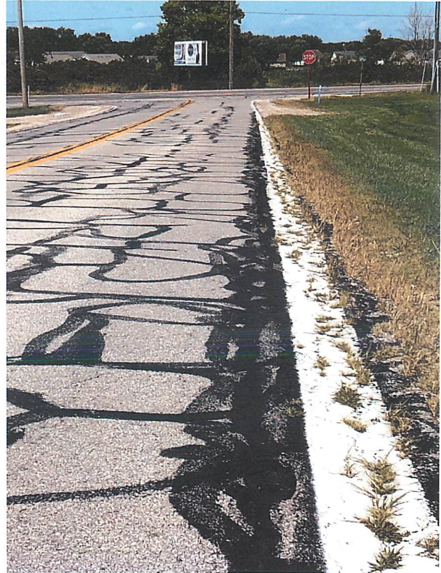
Photo 2 – Edge Failure and Widespread Cracking
