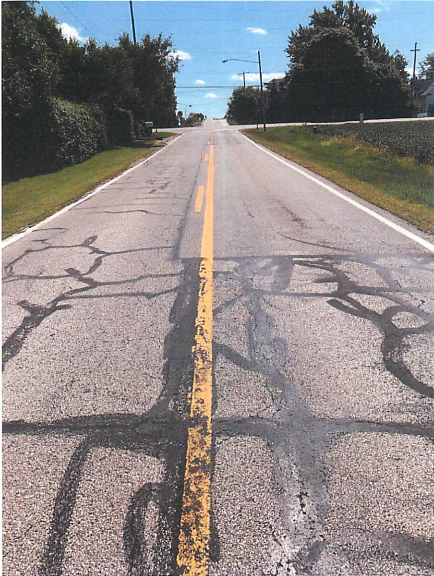
Photo 1 – Widespread Cracking, Patching, Etc.
