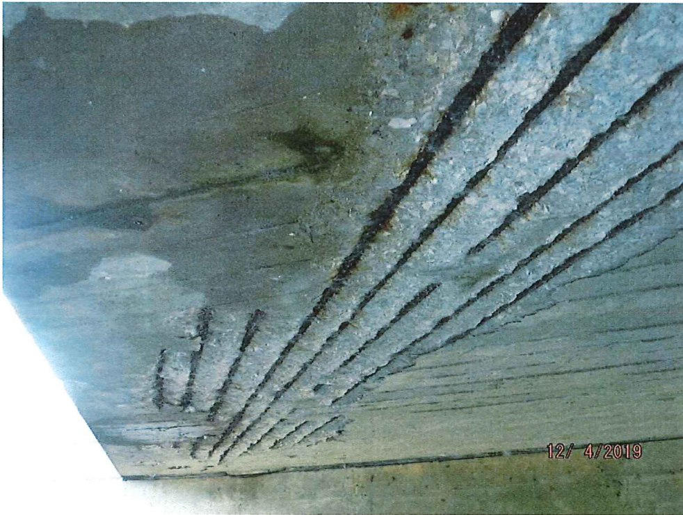
Typical view of Concrete Slab with Exposed Reinforcing Steel
