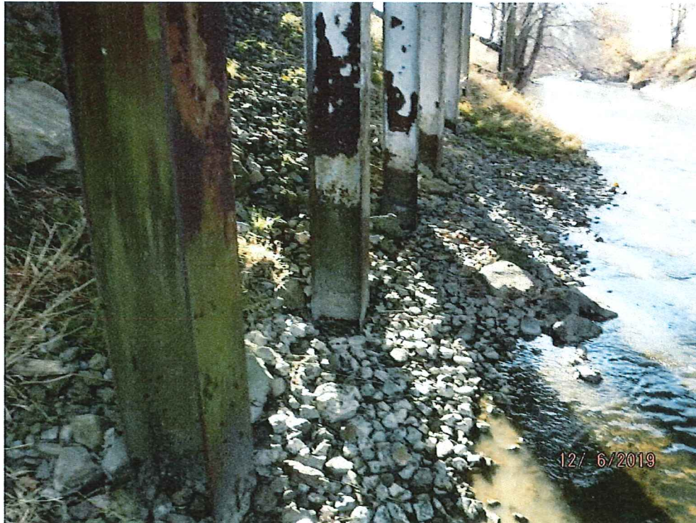
Pier 2 with Exposed Steel H Piles with section loss and pitting at the ground line
