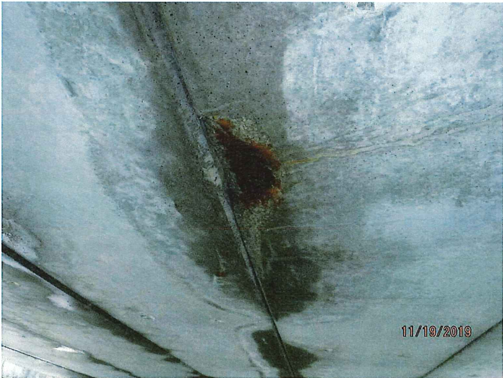
Spall on Beam 3 with exposed prestressing strands near FA
