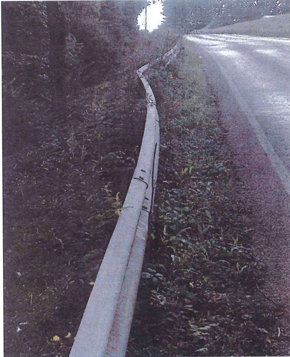
Damaged guardrail from a prior accident. The existing guardrail posts are spaced at 12'6" and are in poor condition.
