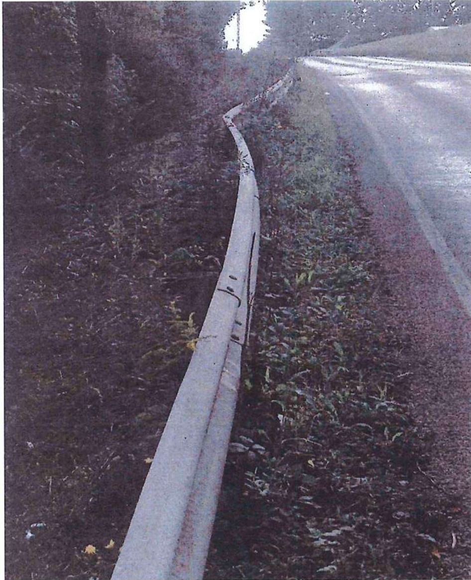
Damaged guardrail from a prior accident. The existing guardrail posts are spaced at 12'6" and are in poor condition.
