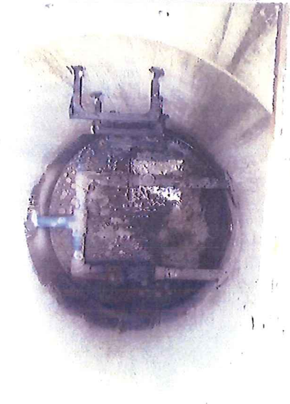
PCI #442 Valve Chamber
