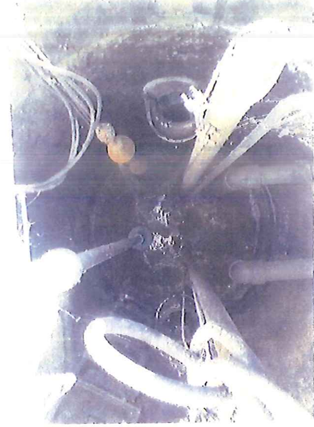
PCI #160 Wet Well
