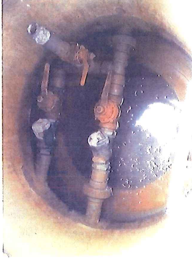
PCI #310 Valve Chamber
