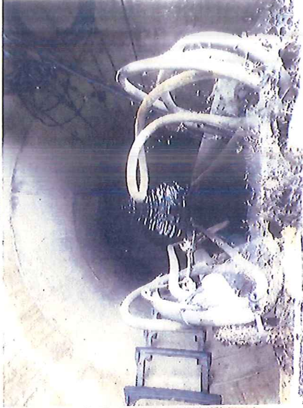
PCI #310 Wet Well
