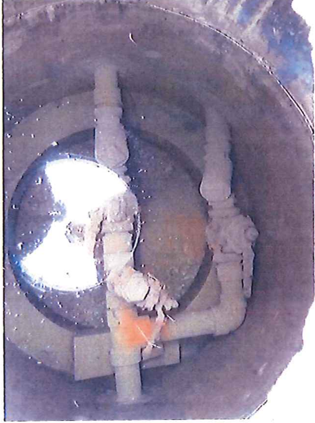
PCI #350 Valve Chamber
