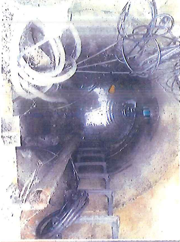
PCI #210 Wet Well
