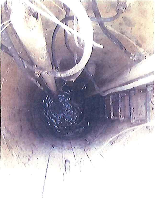
PCI #270 Wet Well
