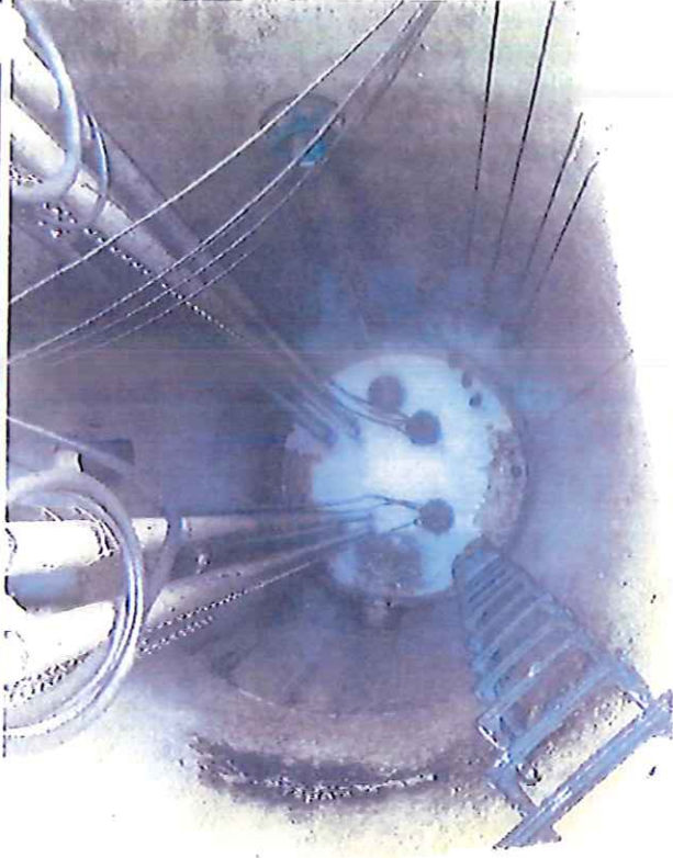
PCI #437 Wet Well
