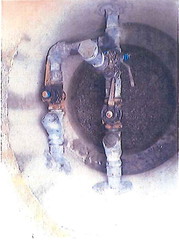
PCI #210 Valve Chamber
