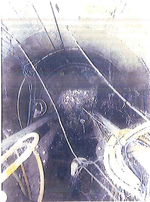
PCI #200 Wet Well
