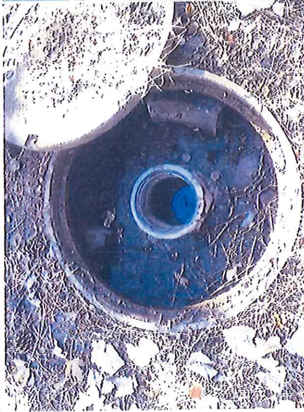
PCI #50 Bypass Discharge
