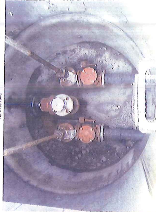
PCI #450 Valve Chamber
