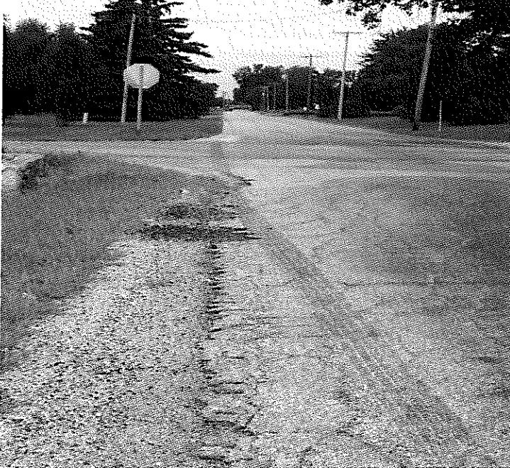
Looking north on Harris Road. The pavement is cracking and chipped.
