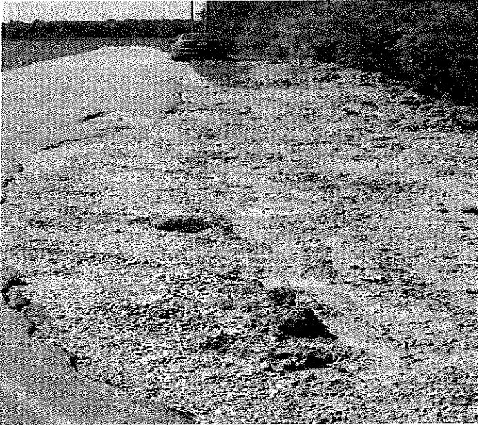
Looking west on Weichman Rd. The pavement is deteriorating and has been replaced with stone.
