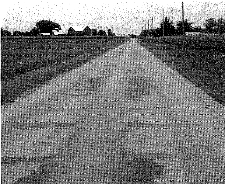
Looking south on Harris Road. There is wheel rutting across the road.
