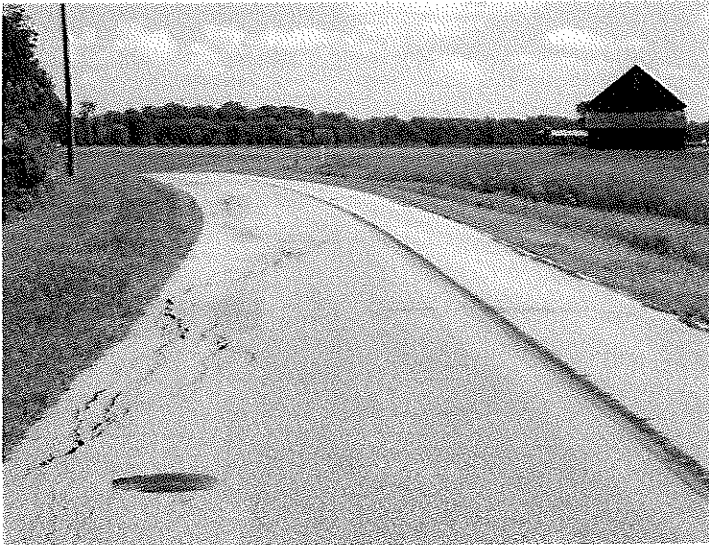
Looking east on Weichman Rd. The pavement is cracking and there is wheel rutting.
