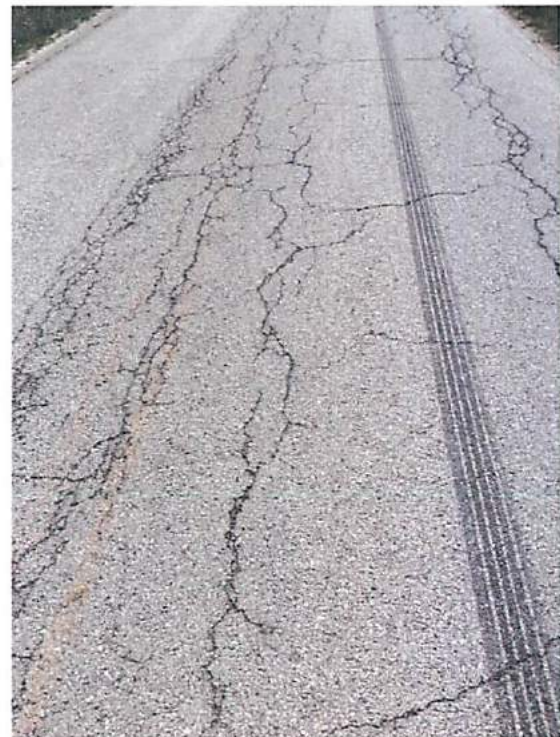
Photos 1, 2, 3, & 4 – Widespread Longitudinal and Map Cracking
