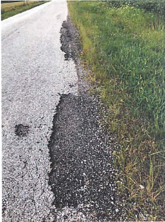
Photo 7 – Potholes Forming at Edges
