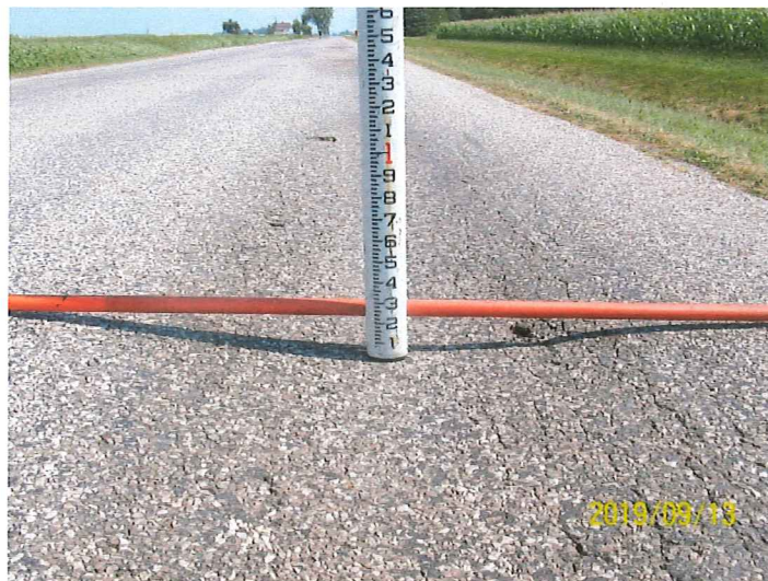
TR-162 Crane Township rut on east bound lane west of CR-87
