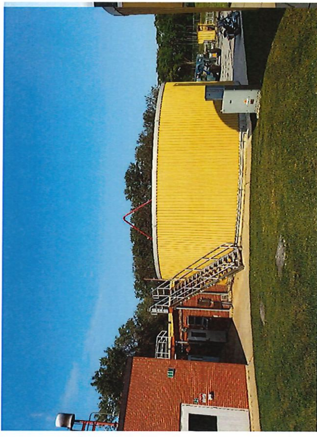
Stairs to Rooftop, no safety railing on roof
