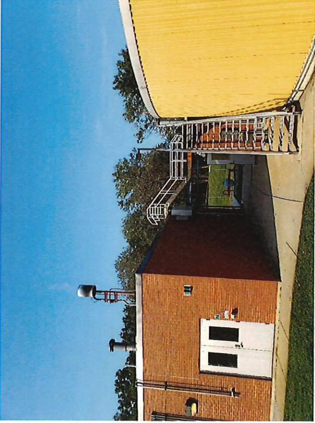
Location of Flare on top of Building, flare installed in 1989
