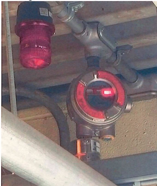
Figure 1 – Gas Monitor and Alarm Beacon
