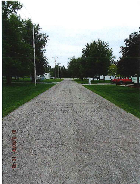
North Oak Street (Between State Route 18 and East Elm Street) - Various locations of cracks and patches
