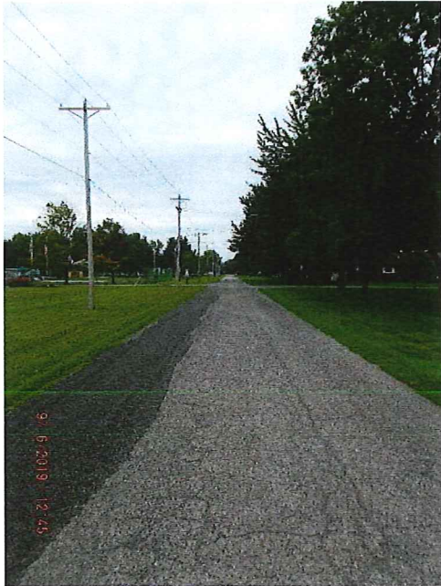
North Oak Street (Between East Elm Street and construction joint at curve) - Various locations of cracks and patches
