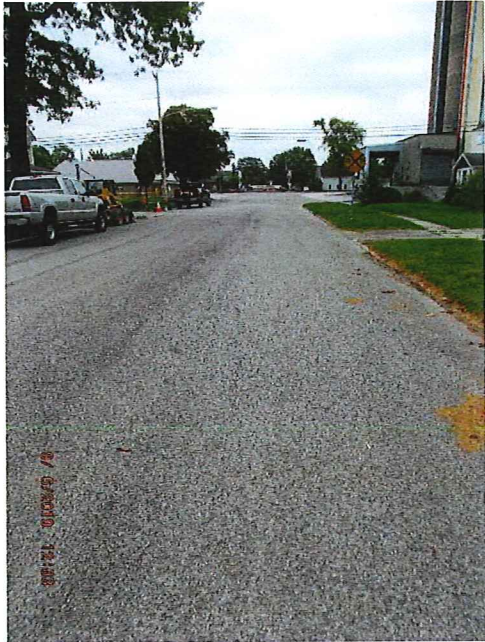
West Maple Street – Various locations of cracks and patches
