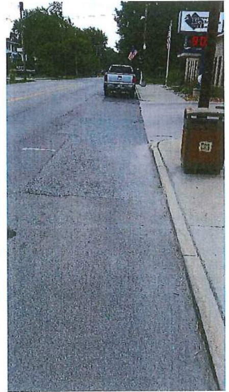
Multiple Patches from Repairs
