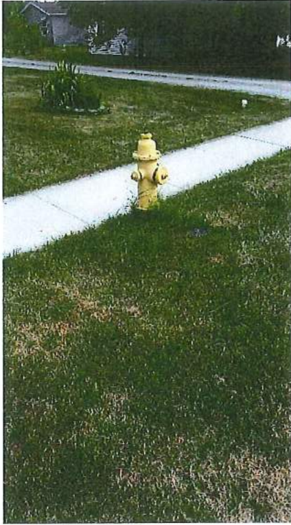
Hydrant to Replace
