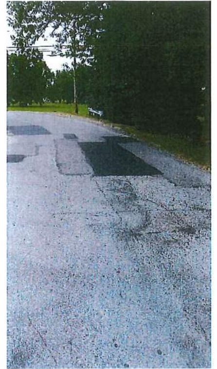
Multiple Patches from Repairs
