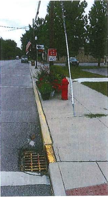
Hydrant to Replace
