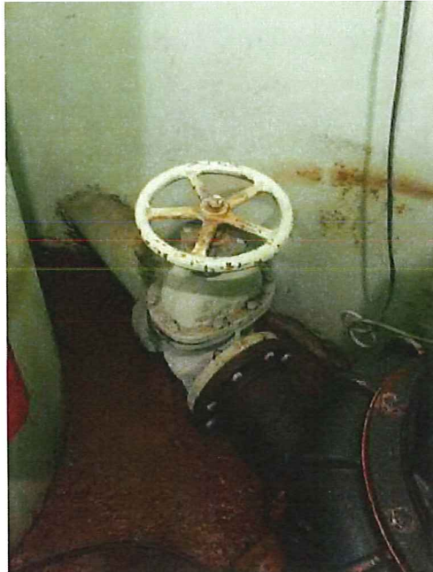
Figure 5– Inside Dry Well at Pump Station #1
