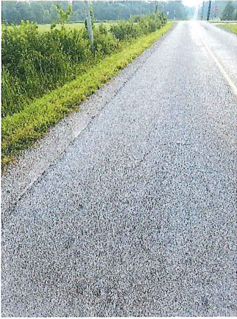
Road R – Various locations of cracks, patches, and close approximately of the ditch along road
