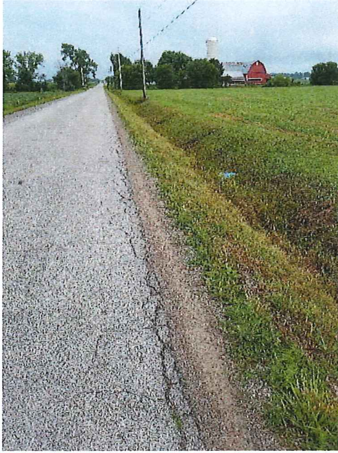
Road S – Various locations of cracks, patches, and close approximately of the ditch along road
