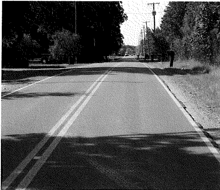
Looking South on Christy. The edge of pavement is cracking and there is wheel rutting across the road.
