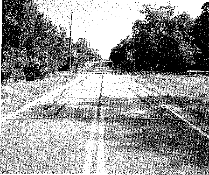
Looking North on Christy. There is wheel rutting across the road.
