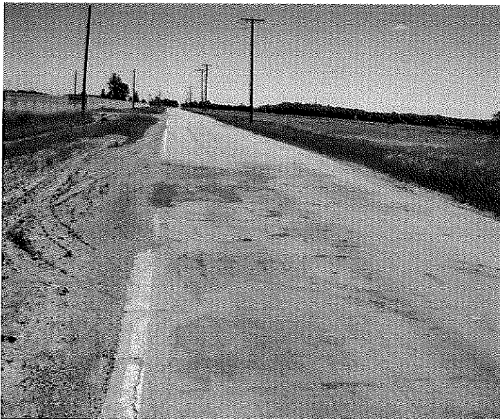
Looking east on Banner School Road. The paving is cracking and chipped.
