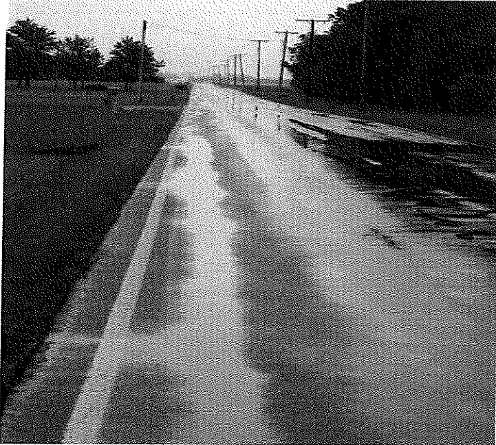
Looking east on Banner School Road. There is wheel rutting.
