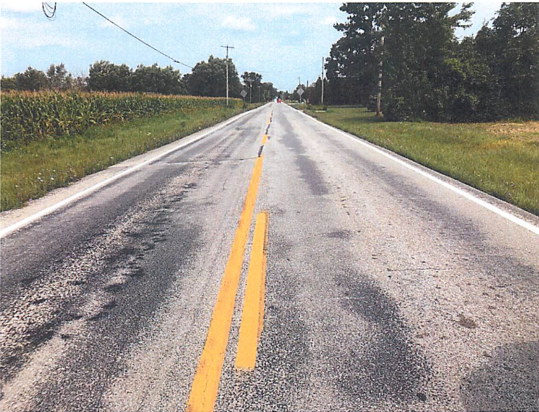
Photos 3 & 4 – Extensive Bleeding, Random Cracking, Patching, Rutting, Etc.
