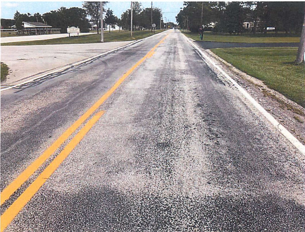
Photos 1 & 2 – Extensive Bleeding, Random Cracking, Patching, Etc.
