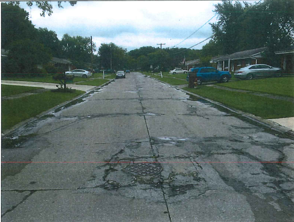
Picture 5 – Maplevue Drive approx. 300' west of intersection with Hollyview Drive. Extensive longitudinal and transverse cracking.
