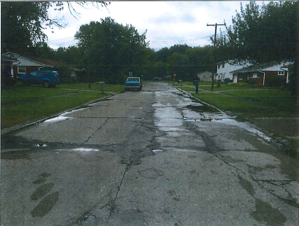
Picture 6 – Maplevue Drive approx. 200' west of intersection with Hollyview Drive. Isolated areas of base failure causing settlement and ponding of water.
