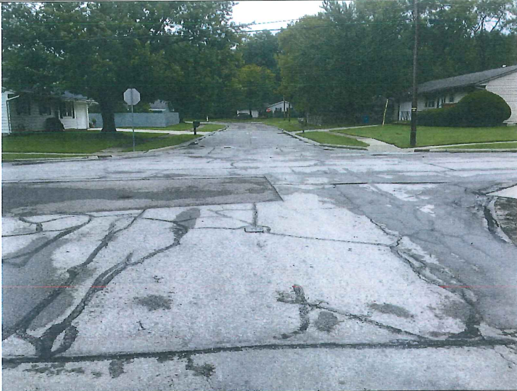
Picture 9 – Mapleview Drive at Hollyview Drive. Transition to asphalt pavement through intersection. Asphalt is in fair condition with map cracking and asphalt settling along concrete gutter.
