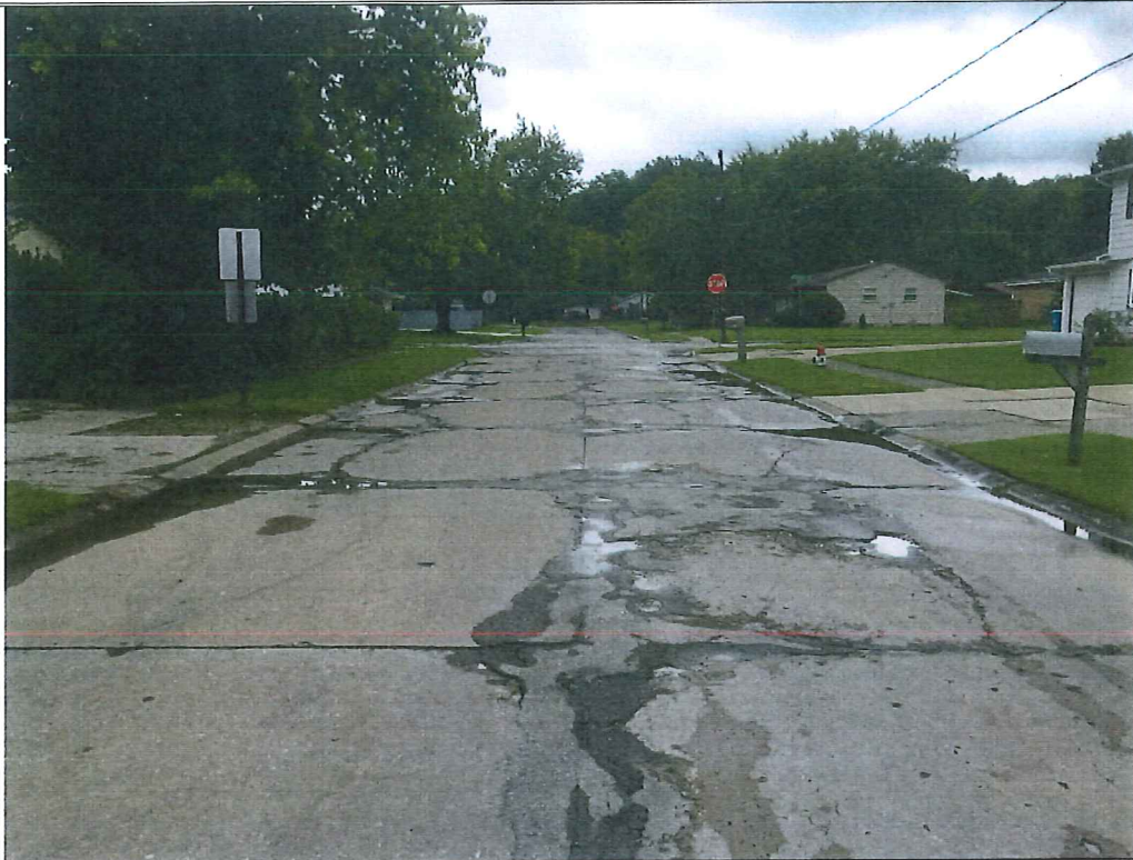
Picture 7 – Mapleview Drive approx. 160' west of intersection with Hollyview Drive. Poor drainage, extensive longitudinal cracking in the middle of concrete slabs. Longitudinal and transverse joint cracking and patches.
