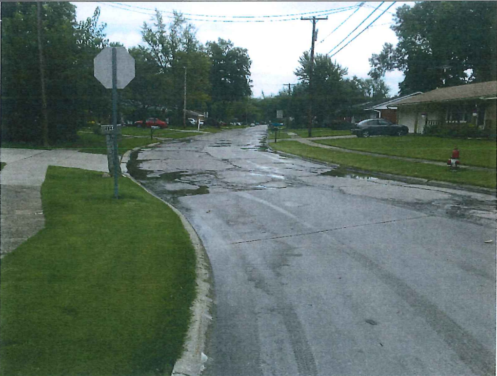
Picture 2 – Mapleview Drive at Forestview Drive. Standing water caused by poor gutter slopes and recent panel replacement. Just east of intersection the roadway transitions to poor rideability and more frequent patching at corners and joints.
