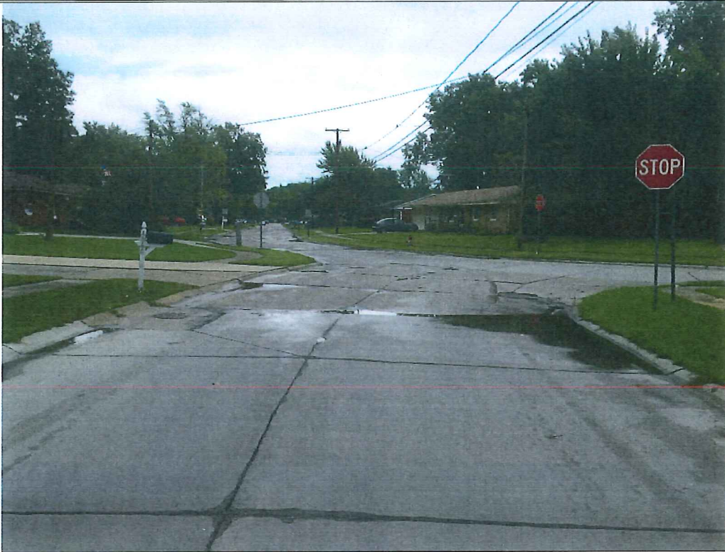
Picture 1 – Mapleview Drive at Forestview Drive. A recent panel replacement is causing a drainage issue.
