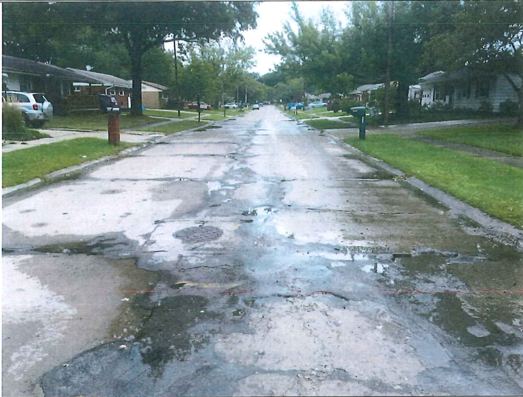
Picture 3 – Mapleview Drive approx. 200' east of intersection with Forestview Drive. Pavement base failure evident on right side of roadway with extensive patching along longitudinal and transverse joints.
