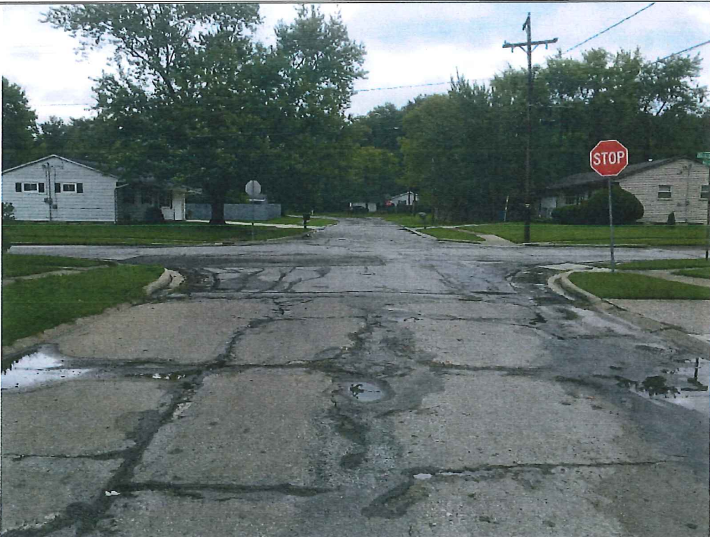
Picture 8 – Mapleview Drive just west of intersection with Hollyview Drive. Poor drainage, extensive longitudinal cracking in the middle of concrete slabs. Longitudinal and transverse joint cracking and patches.
