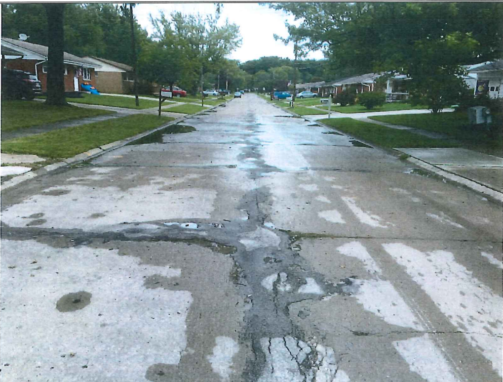
Picture 4 – Mapleview Drive approx. 275' east of intersection with Forestview Drive. Extensive longitudinal/transverse cracking and poor drainage.
