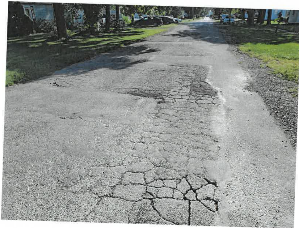
2 – Jackson Street showing failed pavement areas.
