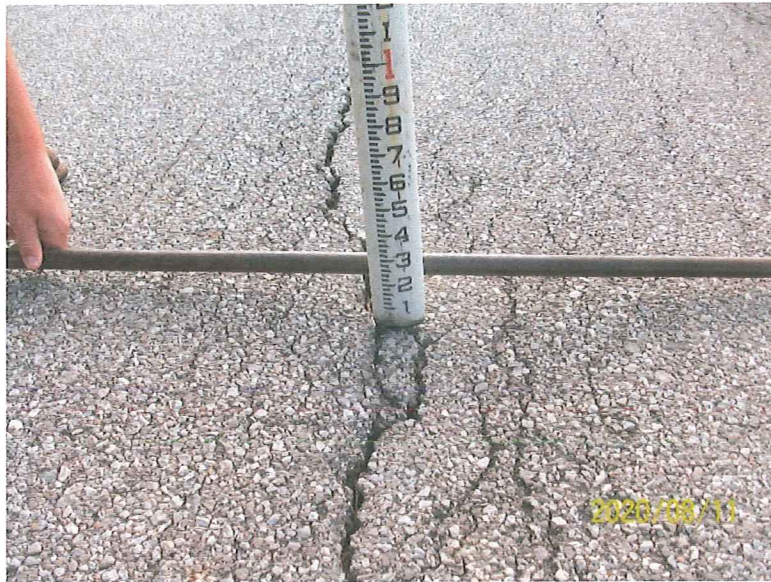
TR-178 rutting east bound lane
