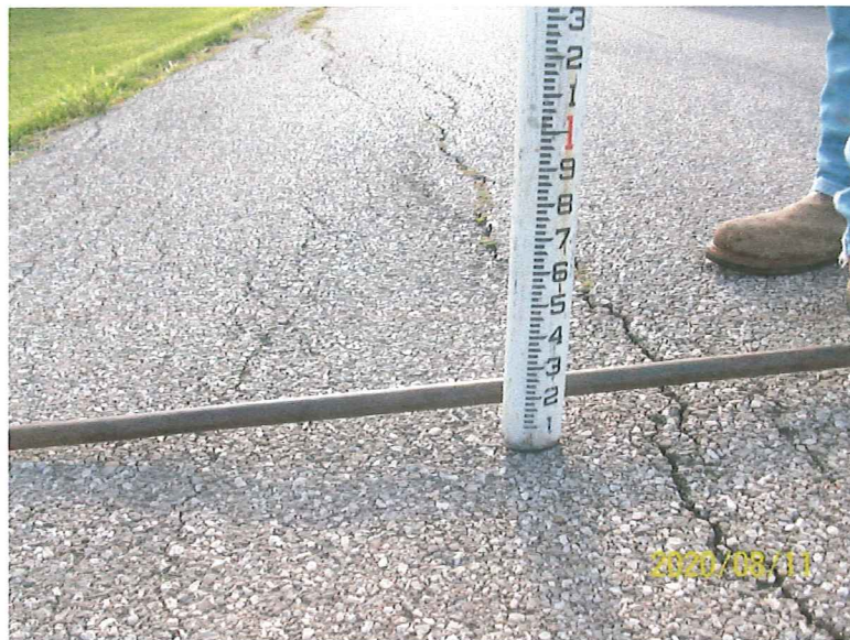
TR-178 longitudinal cracking east bound lane
