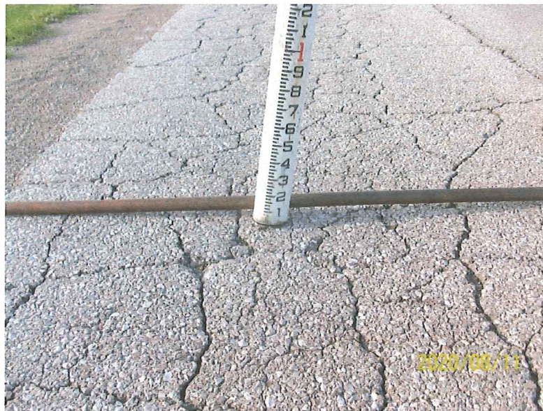
TR-187 rutting south bound lane
