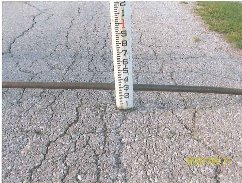
TR-187 rutting north bound lane
