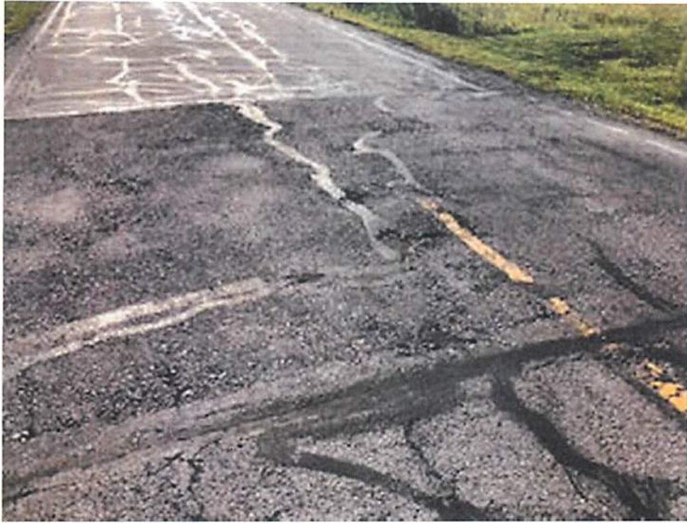
Photo 9 – Failed Patch at Culvert Crossover
