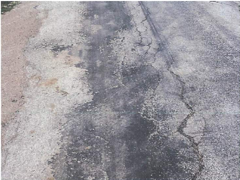
Photo 2 – Failed Edge Repairs
