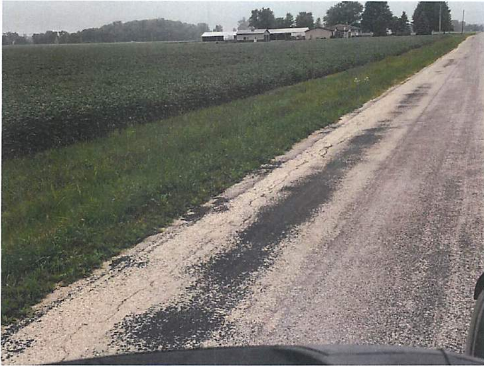
Photo 1 – Edge Failures with Bleeding
