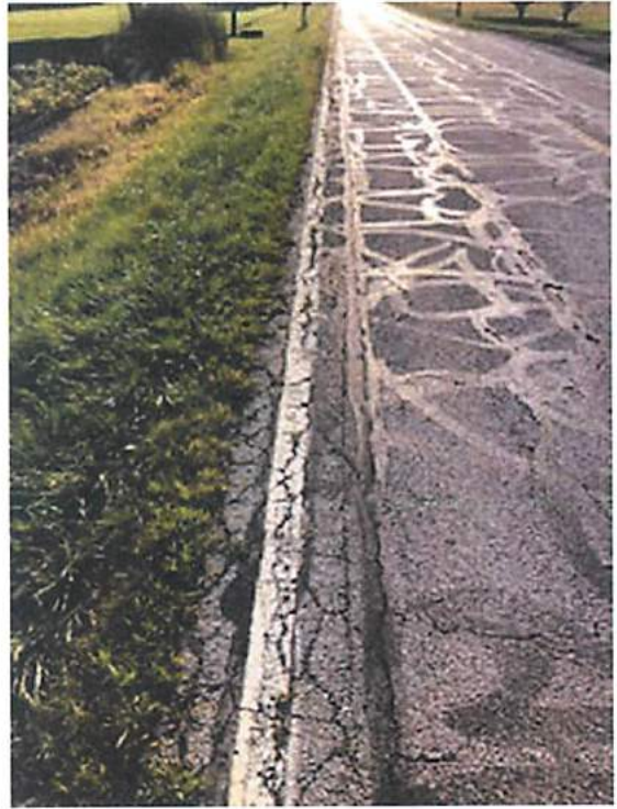
Photos 3 & 4 – Edge Failures
