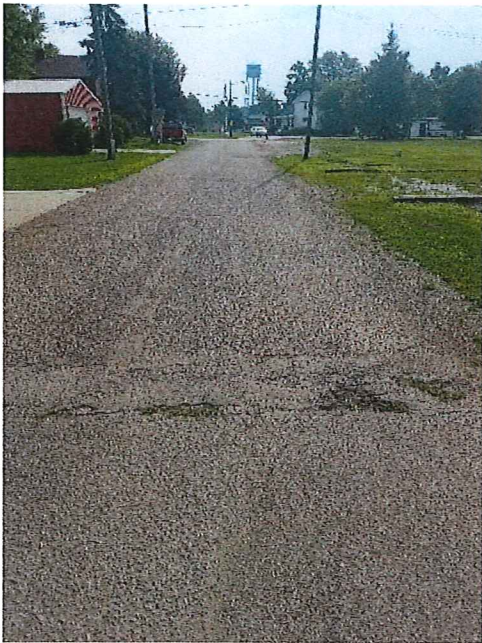
Washington Street – Various locations of cracks, patches, rutting, and pavement loss
