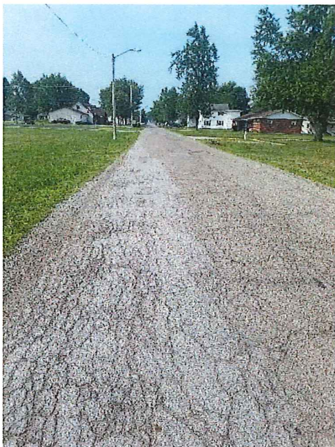
East Street - Various locations of cracks and patches
