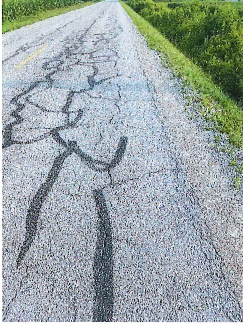
Road 13 – Various locations of cracks and patches
