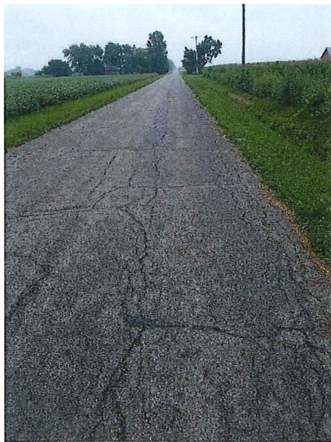
Road 16 - Various locations of cracks and patches
