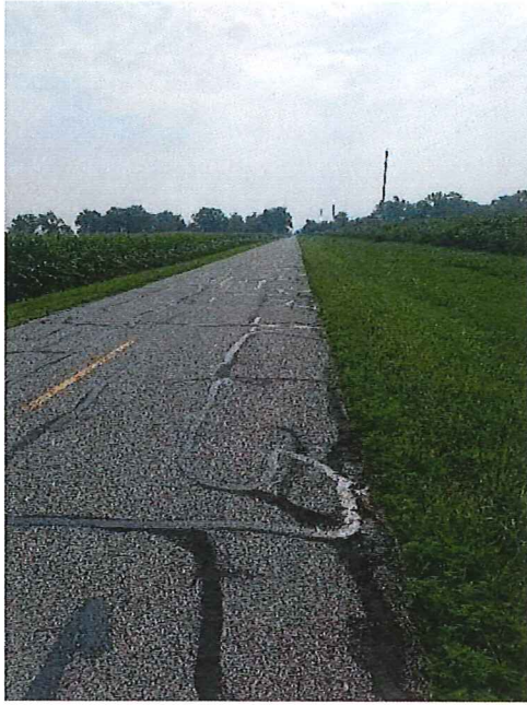
Road K - Various locations of cracks and patches
