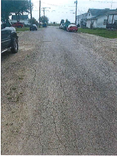
English Street – Various locations of cracks, patches, and rutting
