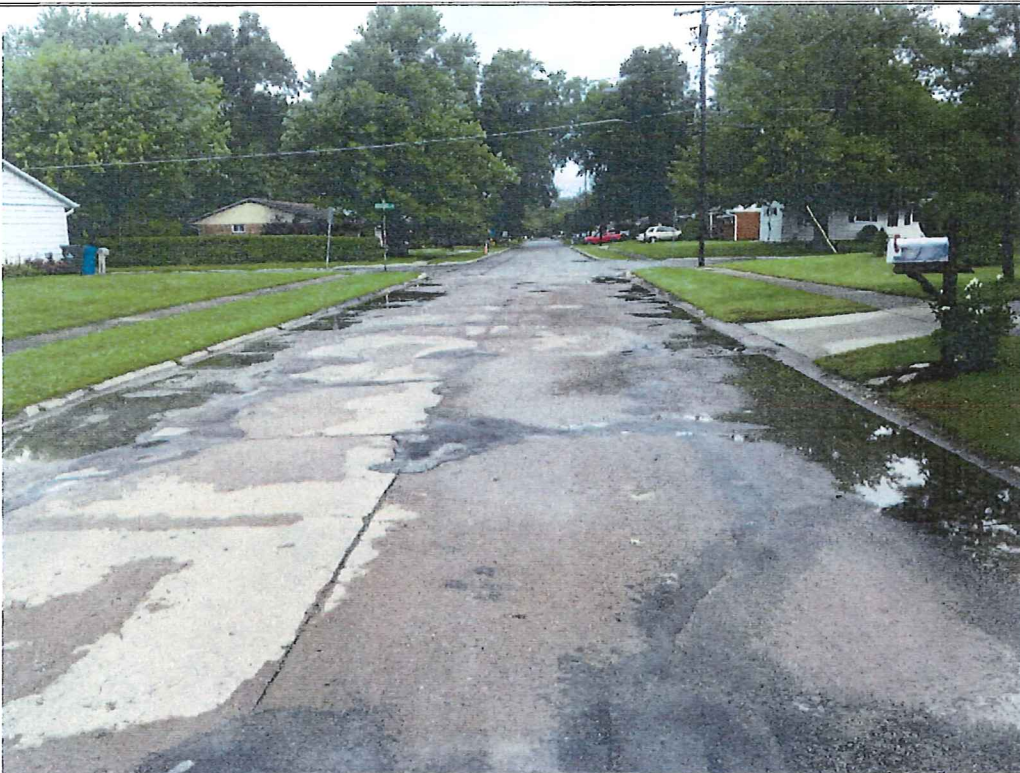
Picture 4 – Hollyview Drive approx. 150' south of intersection with Mapleview Drive. Transverse, longitudinal and diagonal cracking in several panels indicate multiple base failures which are contributing to the drainage issues.
