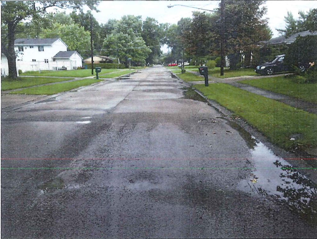
Picture 3 – Hollyview Drive approx. 200' south of intersection with Mapleview Drive. Lack of drainage in this section and longitudinal profile of roadway provides poor rideability at each concrete panel joint causing a noticeable bump.
