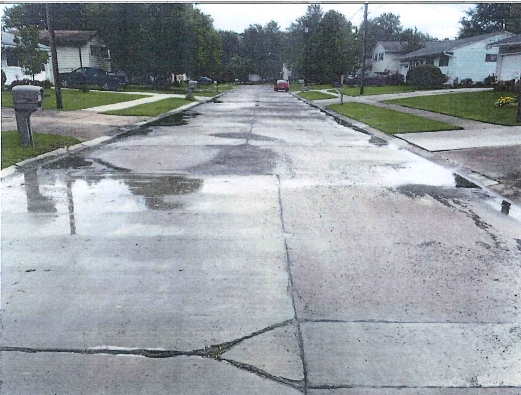
Picture 2 – Hollyview Drive approx. 250' east of Forestview Drive. Shows full depth slab replacement and joint repairs.
