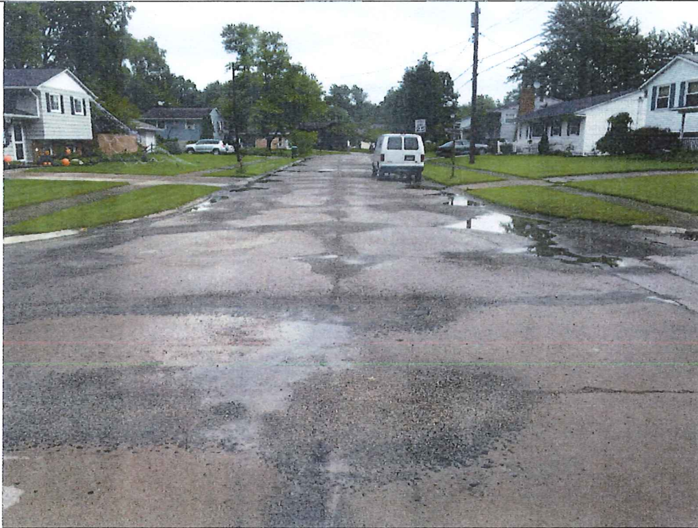
Picture 1 – Hollyview Drive at intersection with Forestview Drive. Concrete pavement is patched at most intersections of longitudinal and lateral joints. Ponding evident due to poor slope and localized failures.
