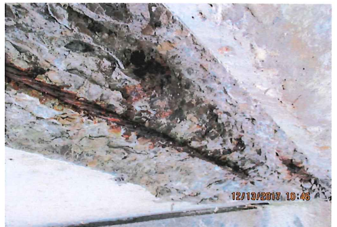
Haber Road Structure V-105. Extensive deterioration of fascia beam concrete. Exposed prestressing strands and reinforcing stirrups. Loss of prestress forces.
