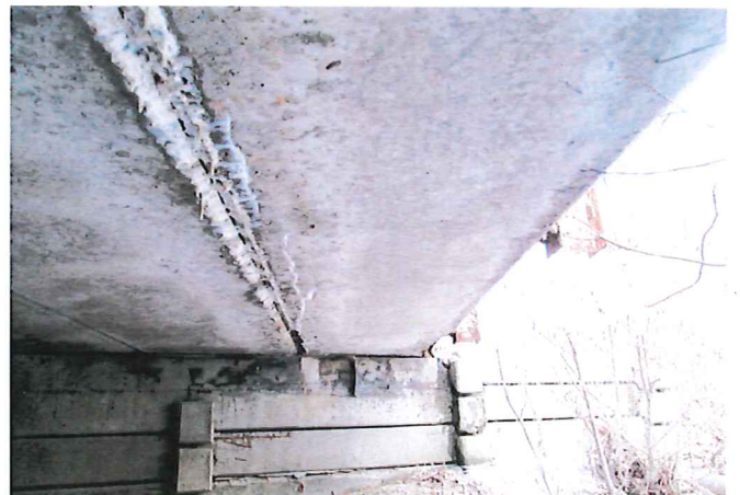
Haber Road Structure V-105. Leakage, saturation, efflorescence, and cracking at beam joints. Probably loss of prestress in strands in vicinity of cracking. These are areas of deteriorated concrete where future spalls are imminent.
