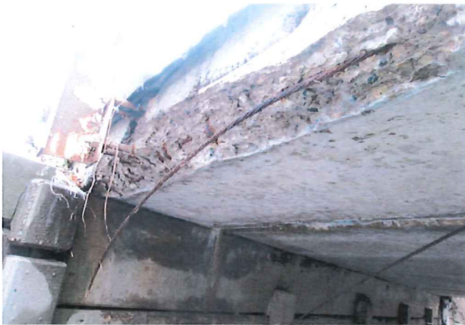
Haber Road Structure V-105. Extensive deterioration of fascia beam concrete. Exposed prestressing strands (note the two strands completely broken and hanging down). Loss of prestress forces.
