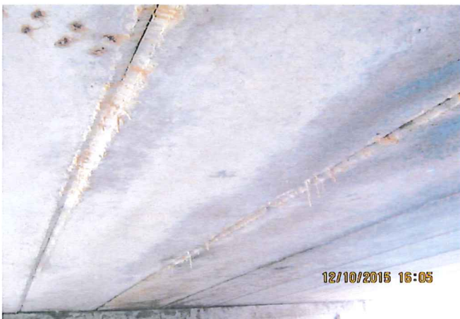
Haber Road Structure V-105. Significant efflorescence on interior structure joints. Saturation of concrete surrounding beam joints.
