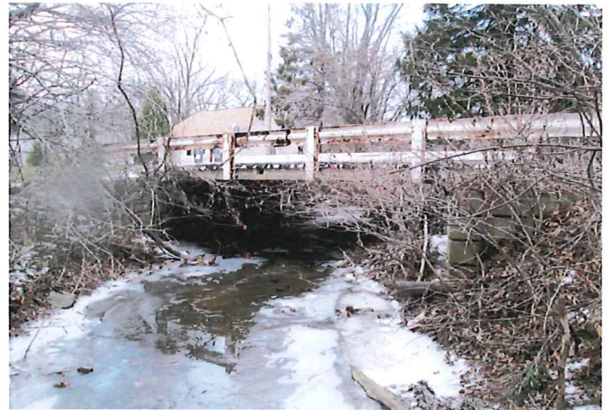
Haber Road Structure V-105. General view of bridge. Bridge is a single-span concrete box beam structure (span 23.92 feet) on built-up precast concrete abutments.
