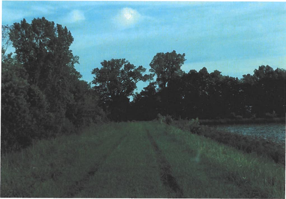
Figure 3 – Ruts in Top of West Dike, Looking North
