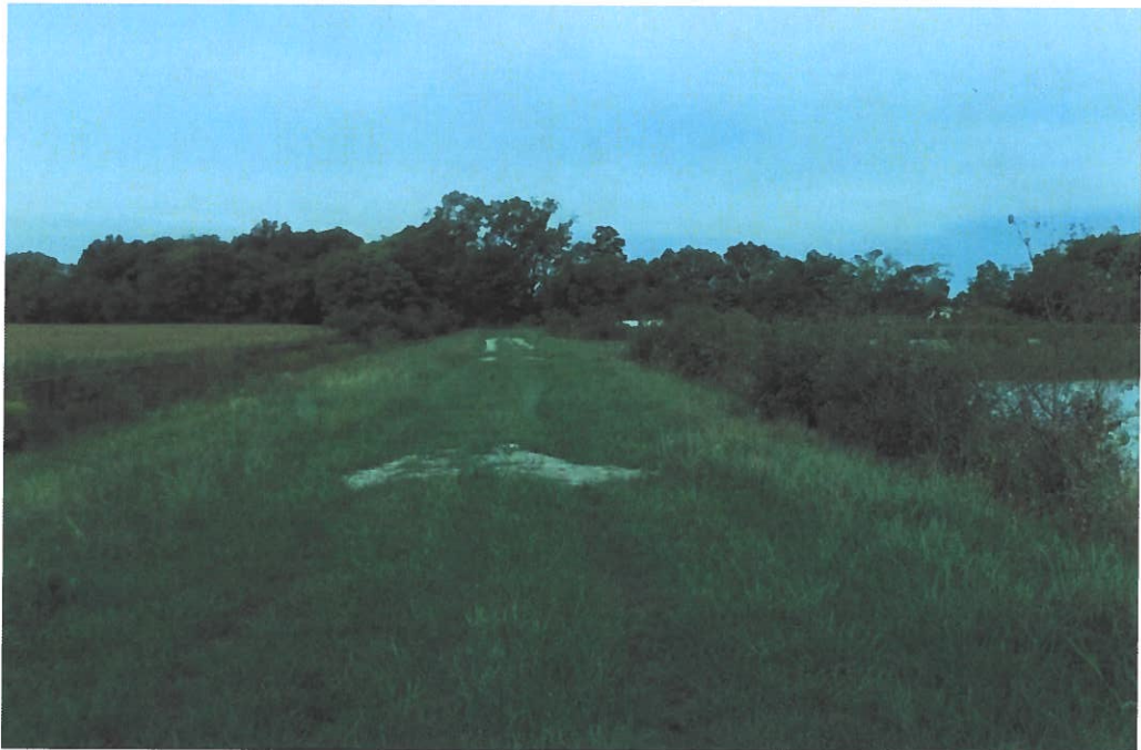
Figure 4 – Ruts in Top of South Dike, Looking West
