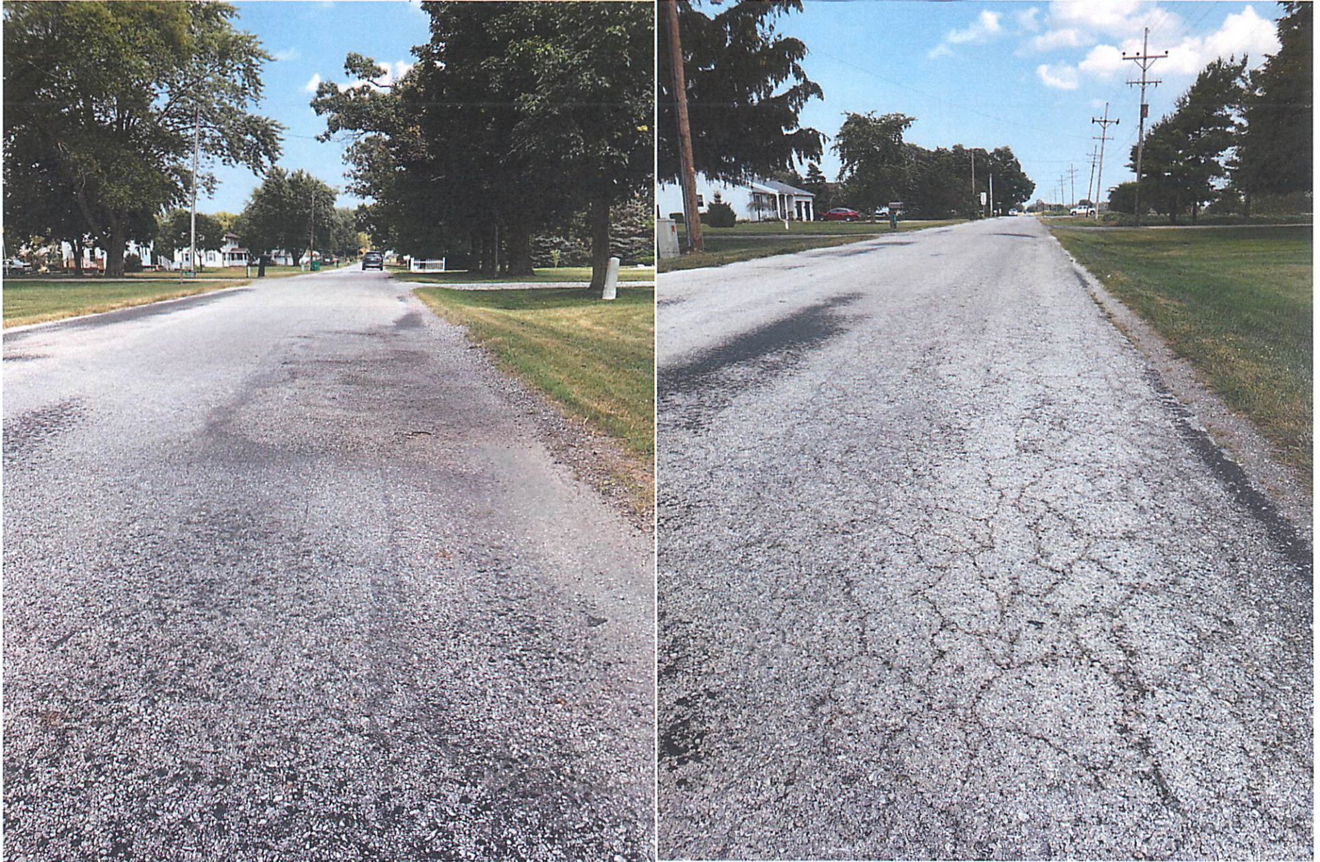
Photos 3 & 4 – Pavement Failures, Raveling & Block Cracking
