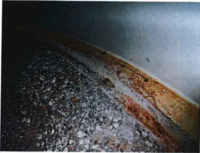
25) Failures on the baseplate.
