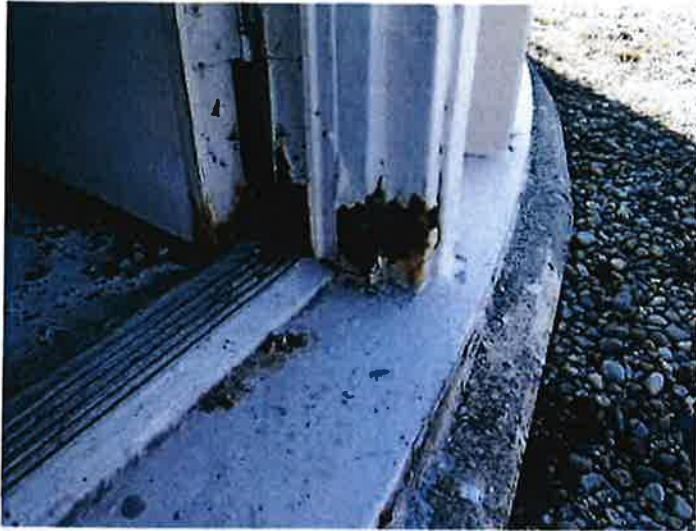
7) There is deterioration on the lower section of the door frame.
