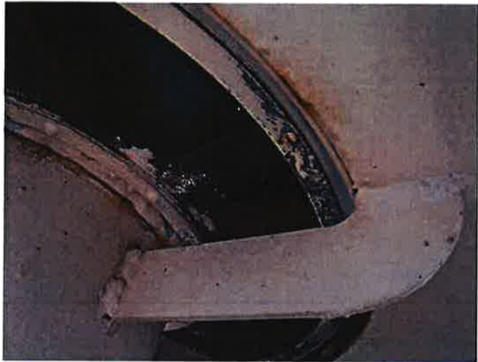
17) The vent screen is in poor condition with large gaps.
