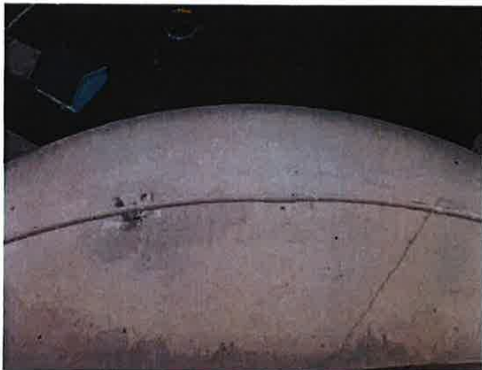
21) Roof painter's railing butt weld is not at stand-off.
