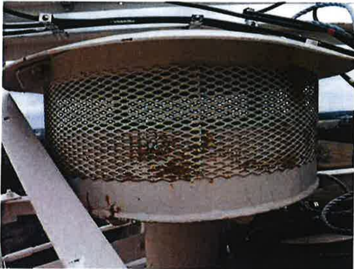
16) The pressure vacuum vent coating is in poor condition.
