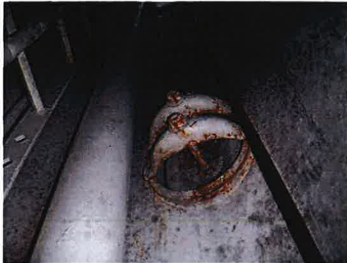
41) The access tube manway is in good condition. The coating is in poor condition.
