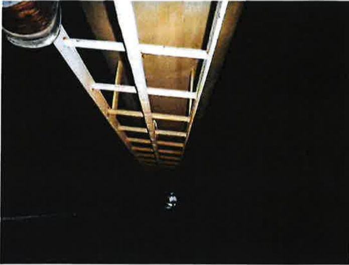
49) The wet interior ladder is in good condition and is equipped with a fall prevention device that operated properly during inspection.
