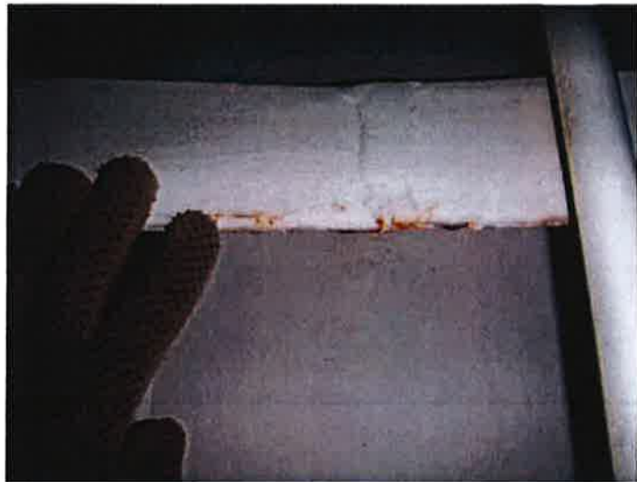
32) Failures on a riser stiffener.
