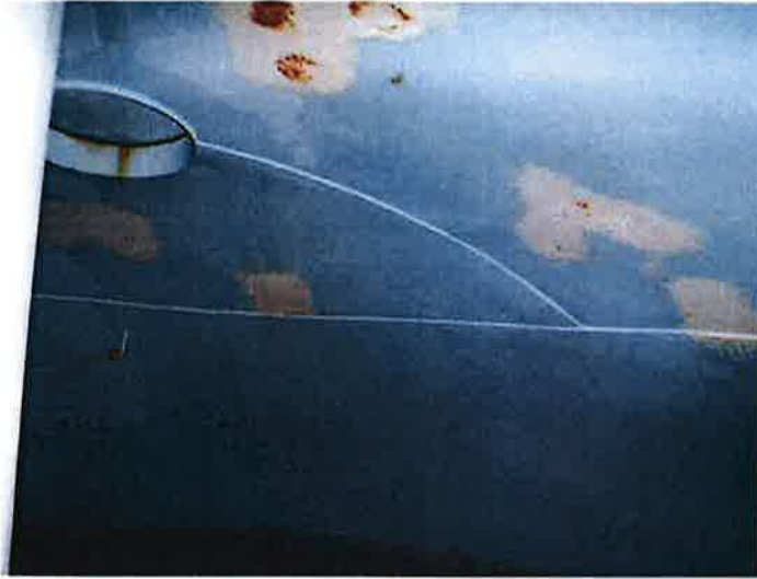
43) The wet interior roof coating is in fair condition with failures at previous spot repairs.
