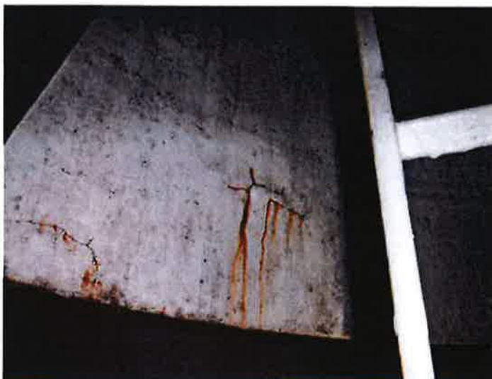
39) Coating failure on the access tube.
