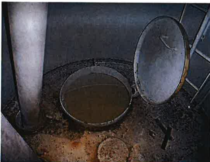
30) Condensate platform opening with hinged cover and handhold. The coating is in poor condition with spot failures to the substrate.
