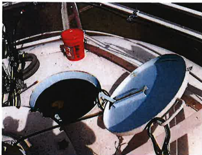
24) The exterior roof hatches are in good condition and operated properly during the inspection.
