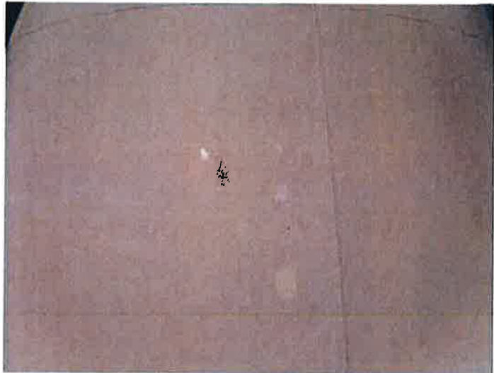
8) Minor coating failures on the basebell.
