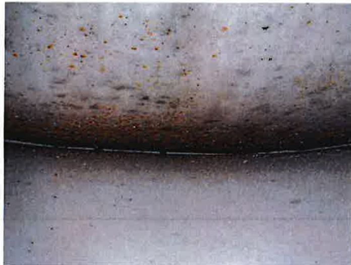
38) Rust bleedthrough on the bowl.
