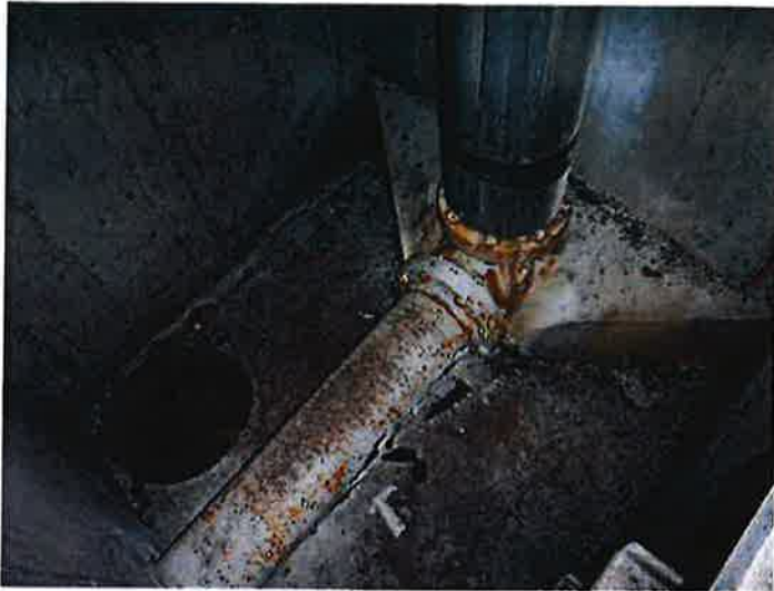
28) The coating on the pit piping is in poor condition.
