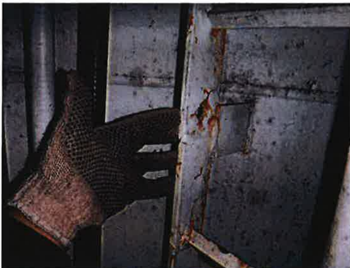
42) Coating failures on the access tube ladder.
