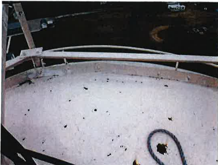
22) The exterior roof coating is in fair condition with spot failures inside the railing.
