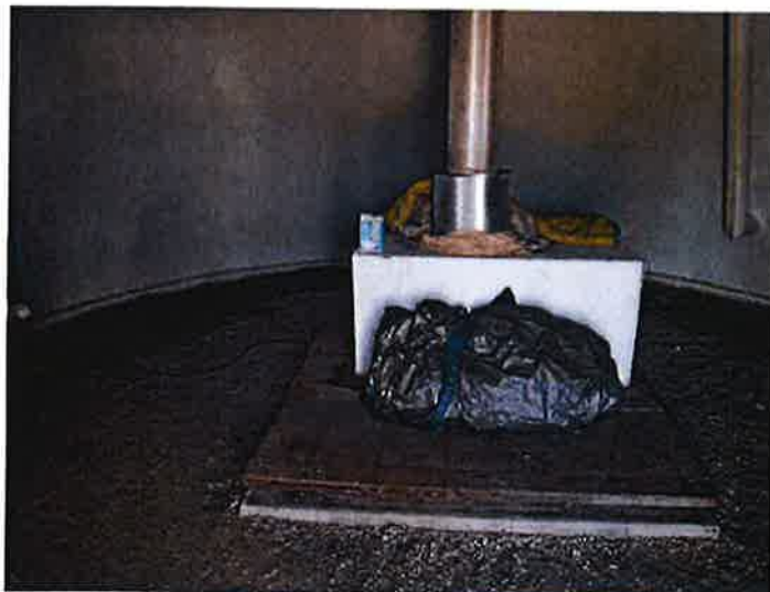
27) The pit piping cover is in good condition.
