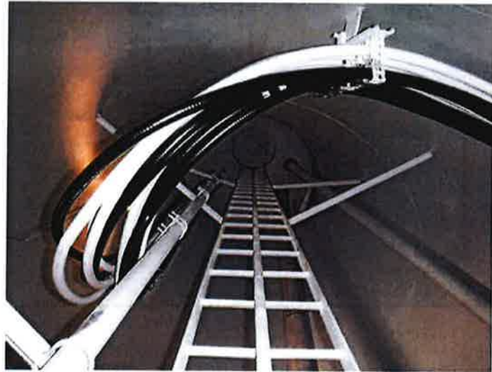
29) The basebell ladder is in good condition and is equipped with a fall prevention device.
