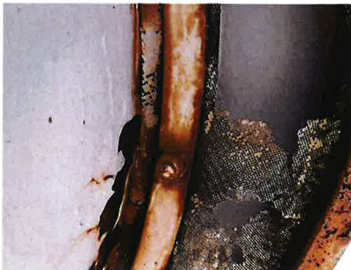
15) Significant deterioration of the access tube air gap screen.
