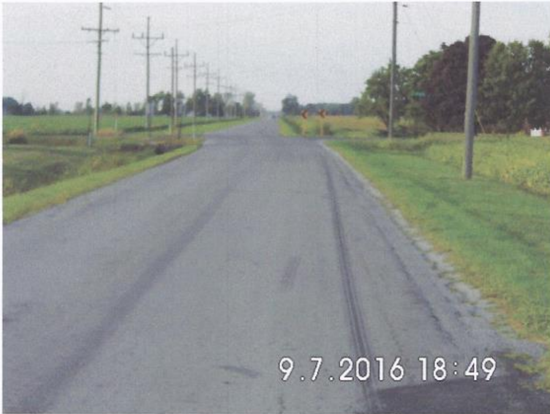
Center of Roadway off-set by approx. 10'
