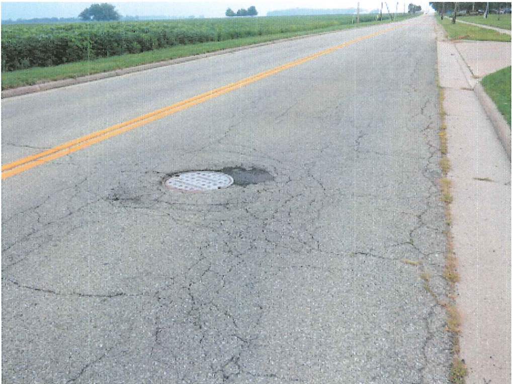
East Lutz Road – Deteriorating Pavement
