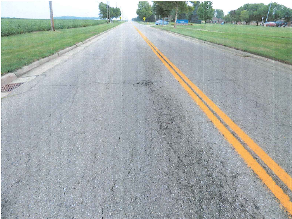
East Lutz Road – Deteriorating Pavement
