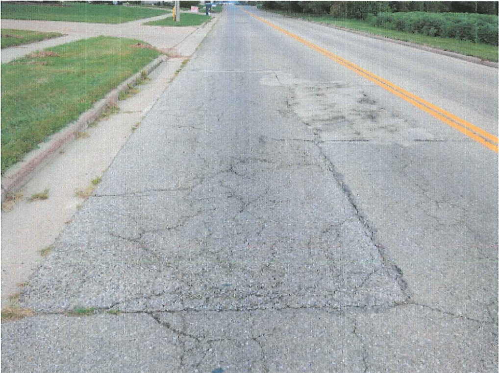
East Lutz Road – Multiple Asphalt Patches from Waterline Repairs
