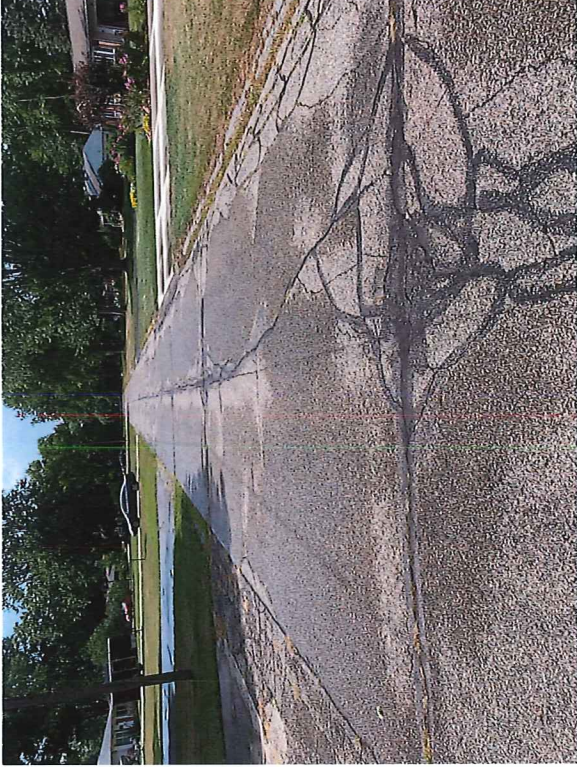
Woodside Drive block cracking along entire road
