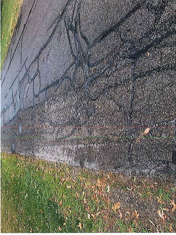
Crestwood Drive pavement cracking and beginning of raveling
