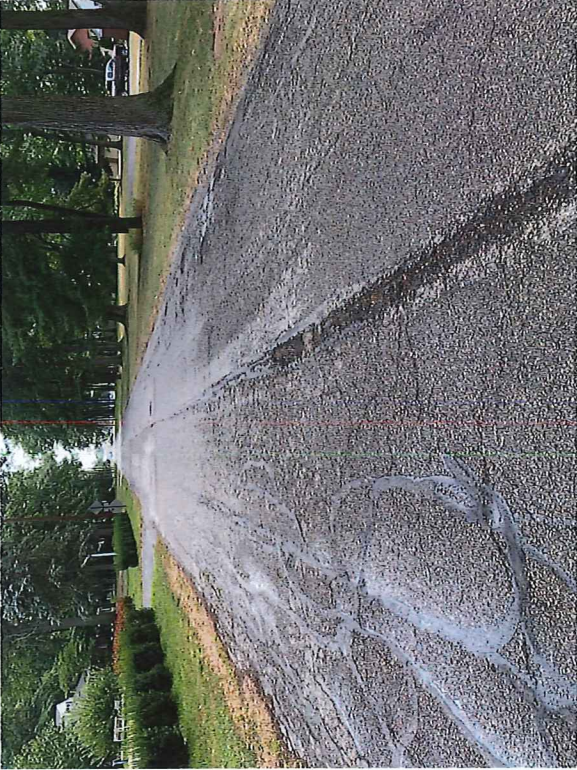
Crestwood Drive failing crack seal on longitudinal cracking
