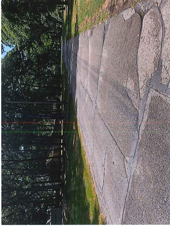
Woodside Drive block cracking
