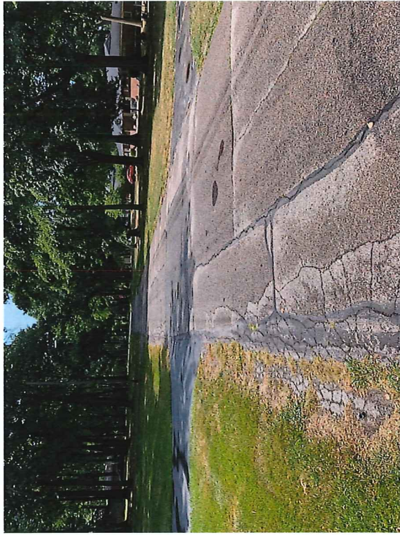
Woodside Drive deteriorated shoulder, edge cracking, & block cracking
