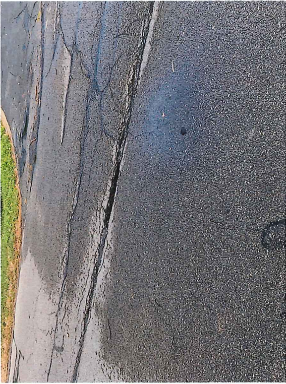
Crestwood Drive longitudinal cracking
