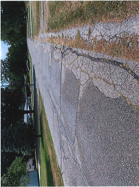
Woodside Drive cracking and deteriorated shoulder
