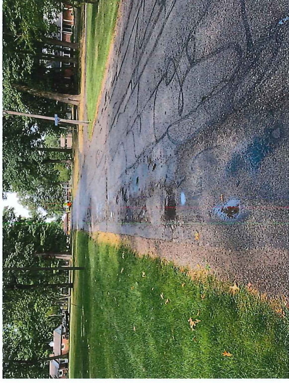
Crestwood Drive potholes holding water after light rain
