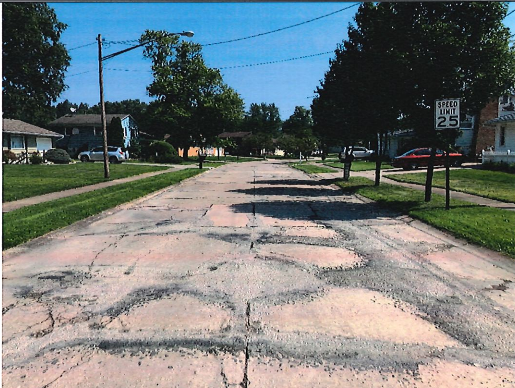
Picture 2 – Hollyview Drive approx. 100' east of Forestview Drive. Extensive patching of panel joints as well as mid-panel longitudinal and transverse cracks.
