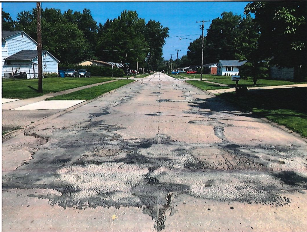
Picture 4 – Hollyview Drive approx. 150' south of Maplevue Drive. Extensive longitudinal cracking and pressure damaged concrete.
