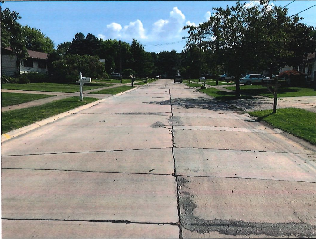
Picture 3 – Hollyview Drive approx. 250' east of Forestview Drive. Mid-block section showing prior joint replacement and multi-panel replacements. This newer section showing signs of D-cracks at corners and deteriorated and open joints.
