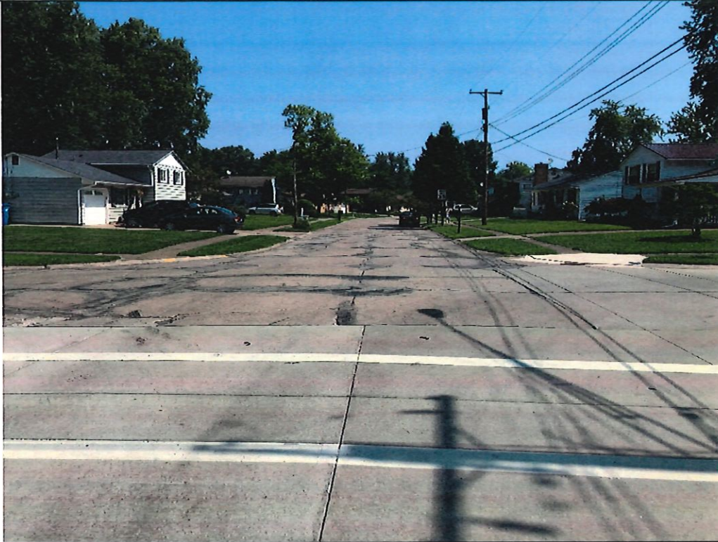
Picture 1 – Hollyview Drive at intersection with Forestview Drive. Extensive patching along longitudinal and transverse joints.
