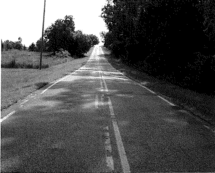
Looking East on Scott Rd. Across the road there is wheel rutting.
