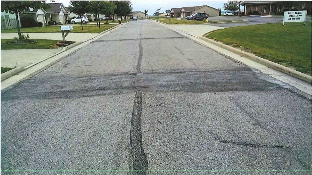
Westfield Drive – Asphalt Spray Patch At Settled Utility Trench
