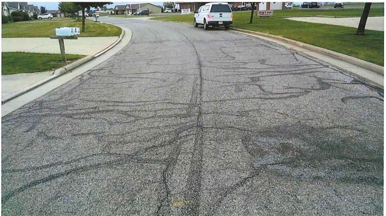
Westfield Drive – Distressed Pavement
