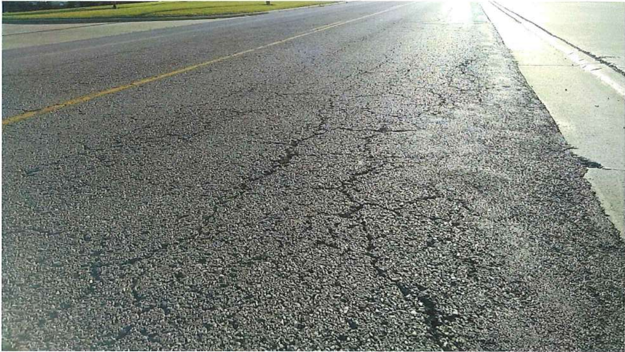
West Barre Road – Surface Raveling & Block Cracking
