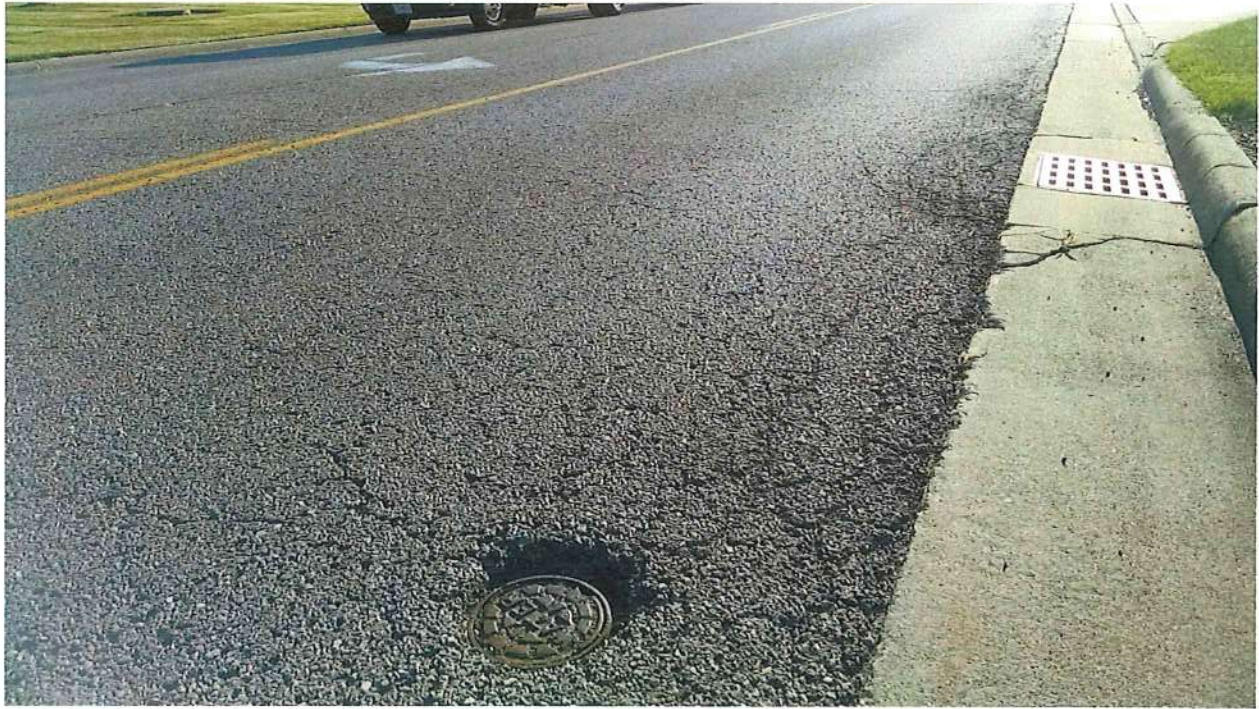
West Barre Road – Distressed Pavement
