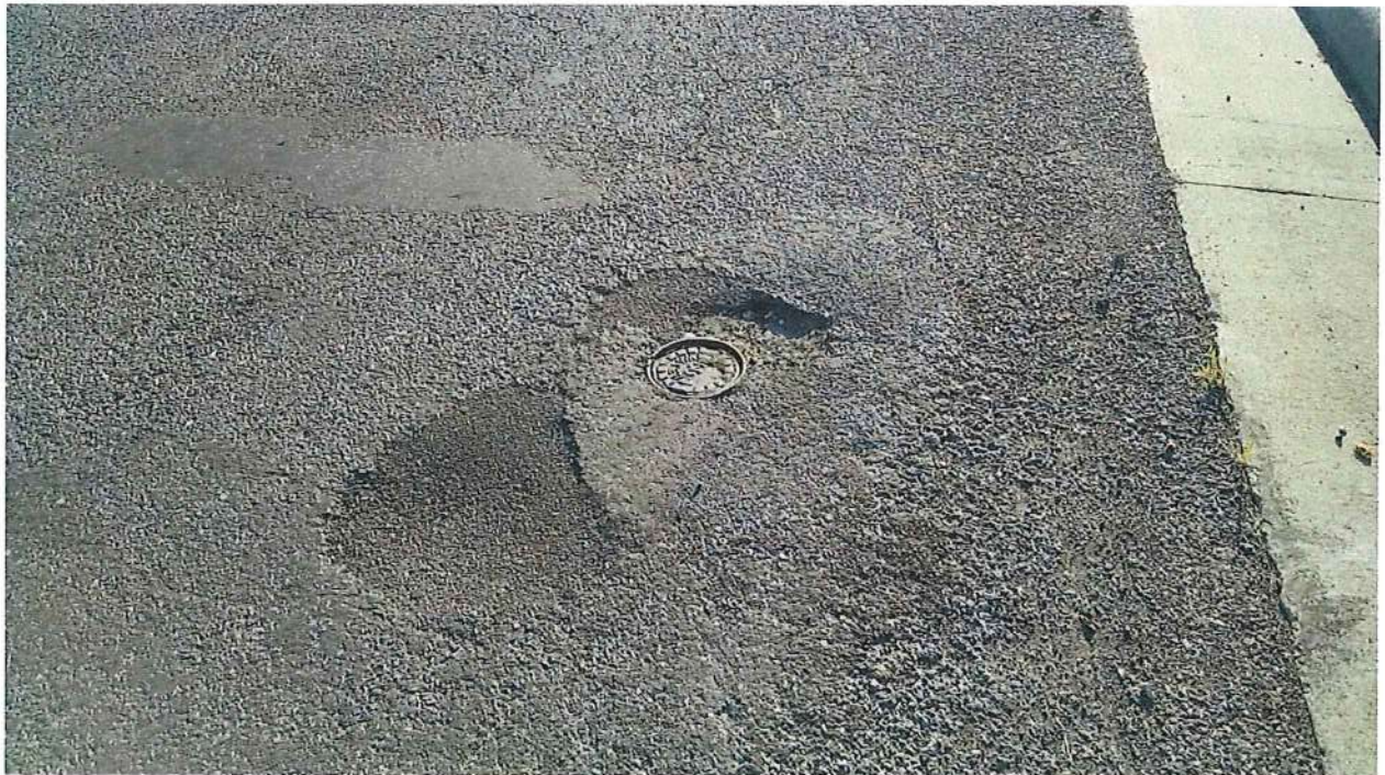
West Barre Road – Loss Of Pavement At Water Valve Box
