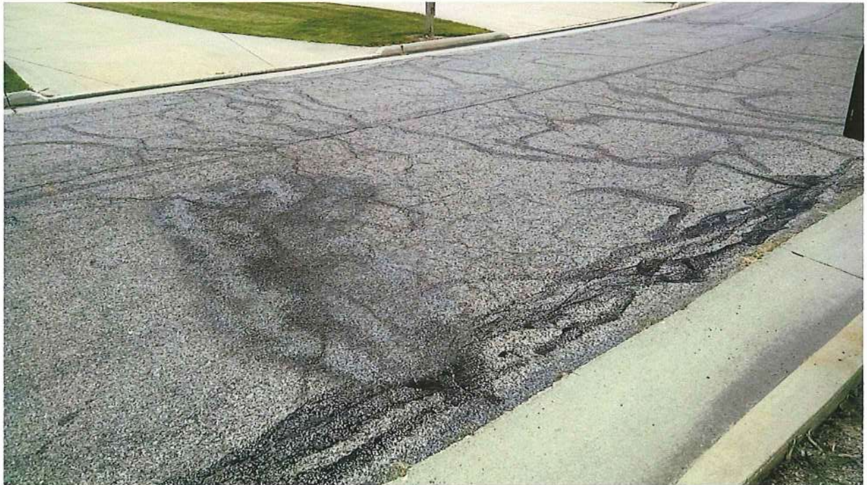
Westfield Drive – Distressed Pavement
