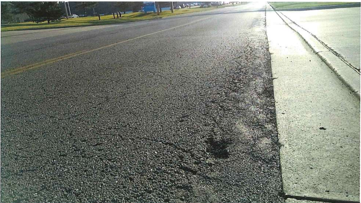
West Barre Road – Asphalt Spray Patch Of Severe Edge Raveling
