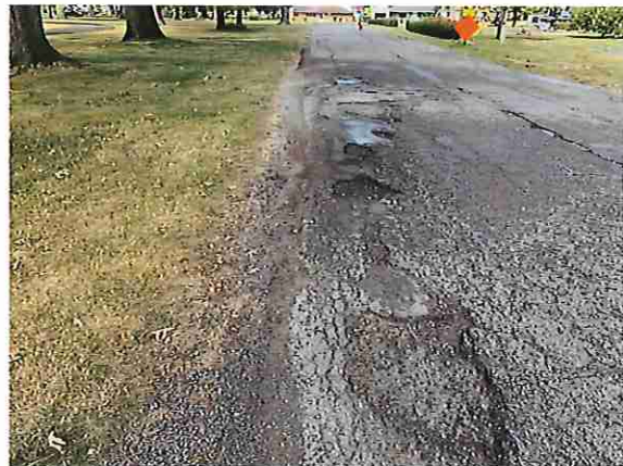
Crestwood Drive potholes and longitudinal cracking
