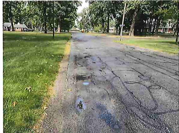
Crestwood Drive potholes holding water after light rain
