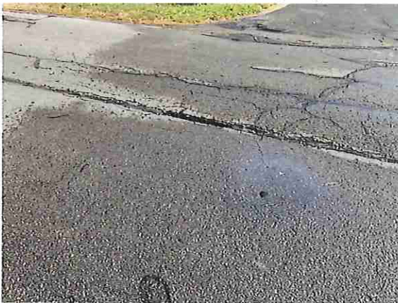
Crestwood Drive longitudinal cracking
