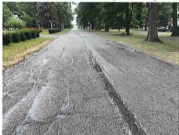
Crestwood Drive failing crack seal on longitudinal cracking
