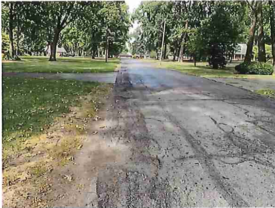
Crestwood Drive potholes, cracking, raveling
