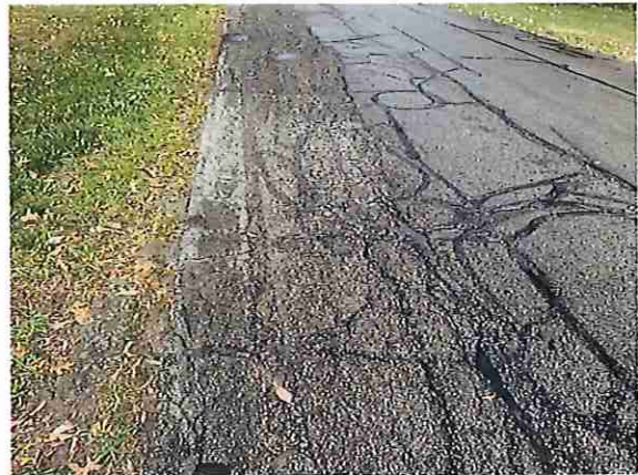
Crestwood Drive pavement cracking and beginning of raveling
