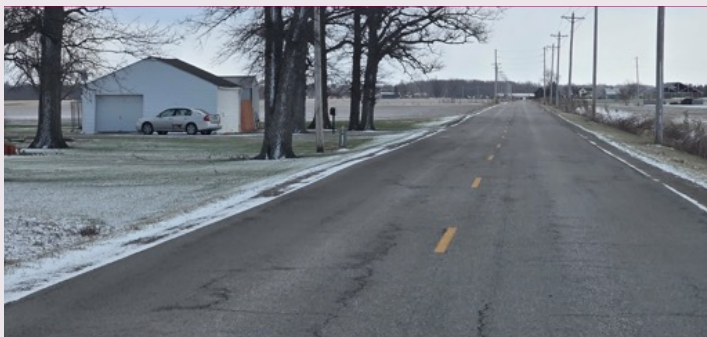
Narrow shoulder and fixed-object exposure on Charloe Trail.
