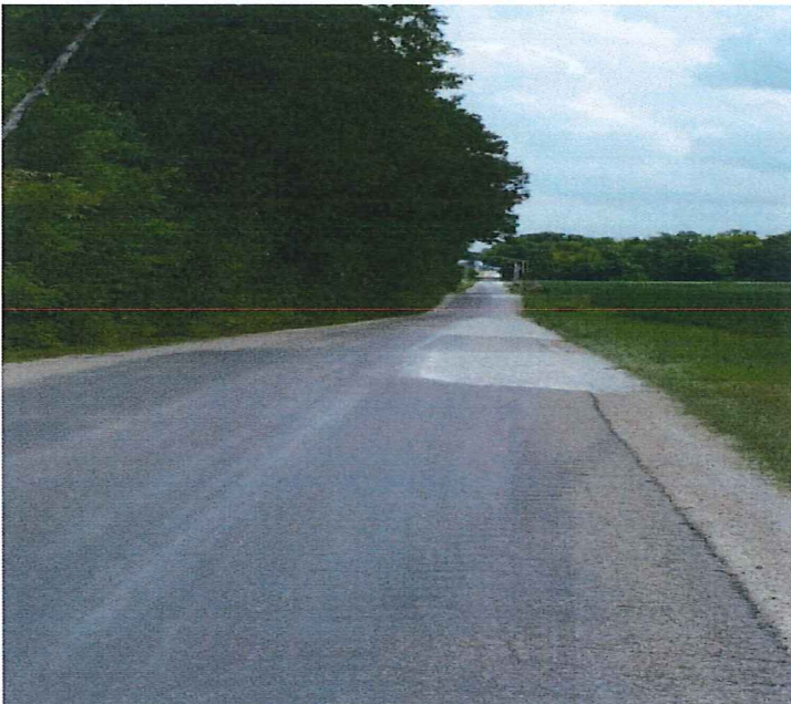
Looking East on Kramer Rd. There is wheel rutting across the road and there are large patched areas.
