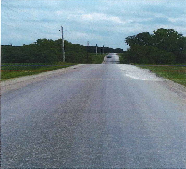
Looking East on Kramer Road. Note large areas that are broken up and patched with stone.
