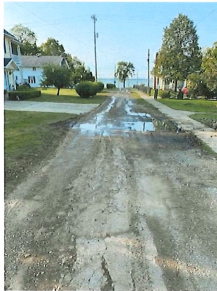
Figure 2: Huntington Lane - Water main leak
