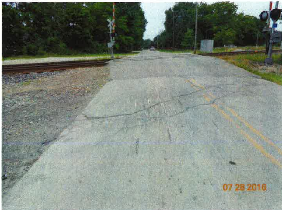
RAILROAD APPROACH WITH VEHICLE SCRAPES ON PAVEMENT
