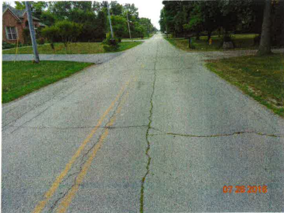
LONGITUDINAL CRACKING IN PAVEMENT
