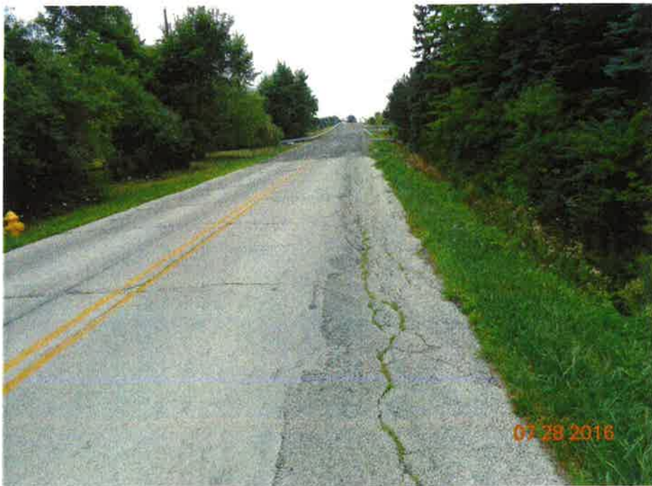
PAVEMENT EDGE SLOUGHING INTO DITCH BANK
