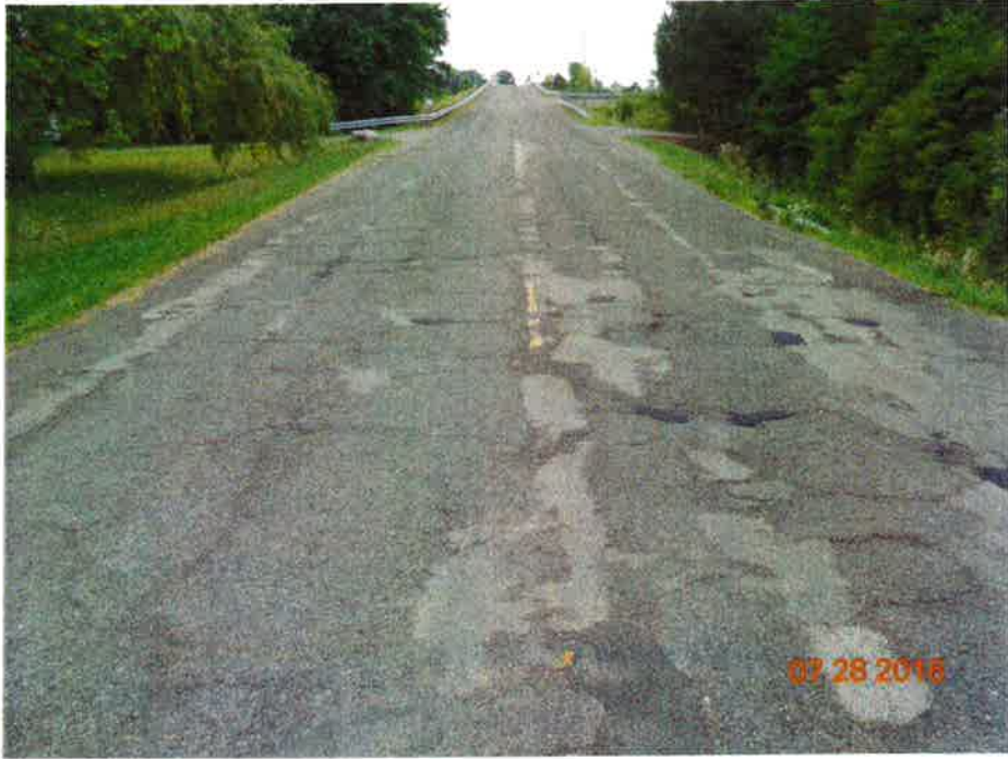
HEAVILY PATCHED PAVEMENT AREAS
