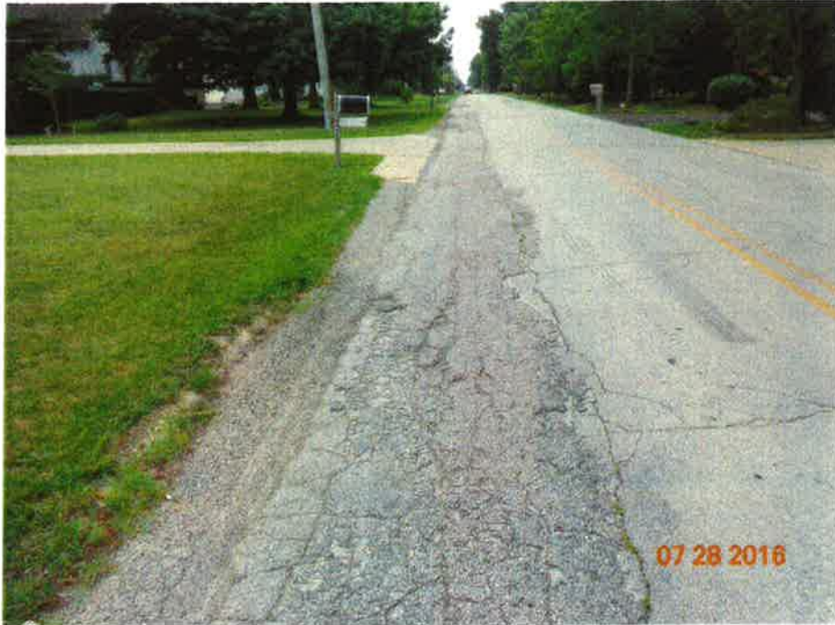
PAVEMENT EDGE DETERIORATION
