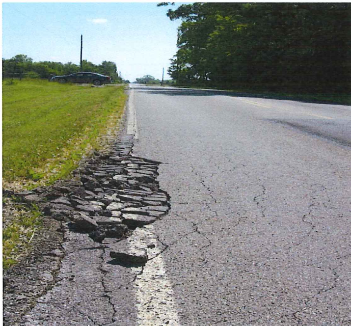
Looking East on Buckskin Rd. The pavement is breaking.
