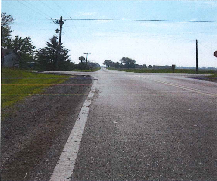
Looking East on Buckskin Rd. Across the road there is wheel rutting.
