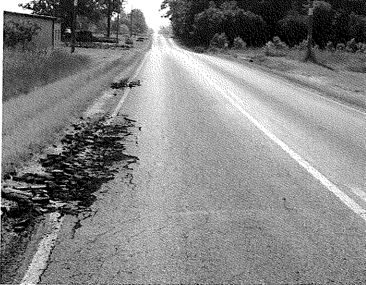
Looking West on Conkle Rd. The pavement is cracked and broken.
