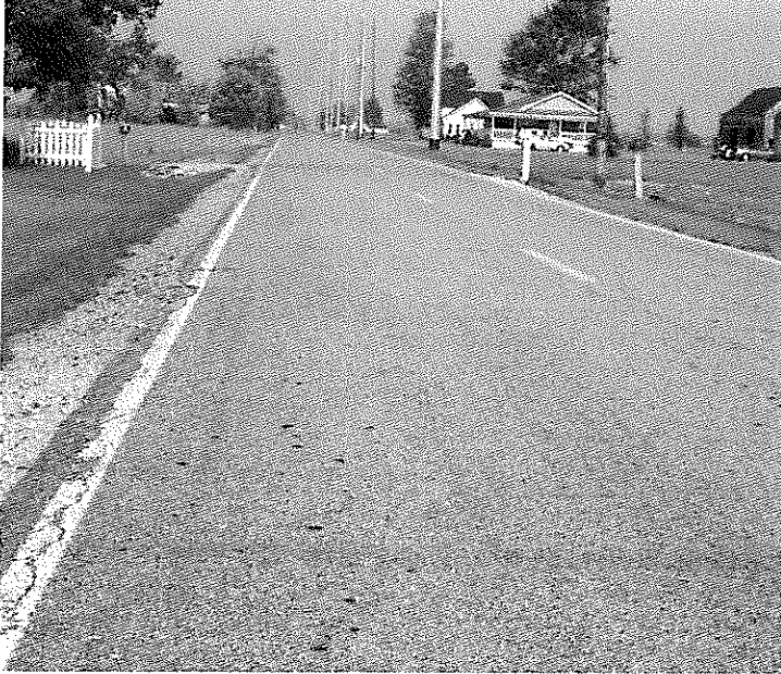
Looking West on Ft St Road. The edge of pavement is cracking.
