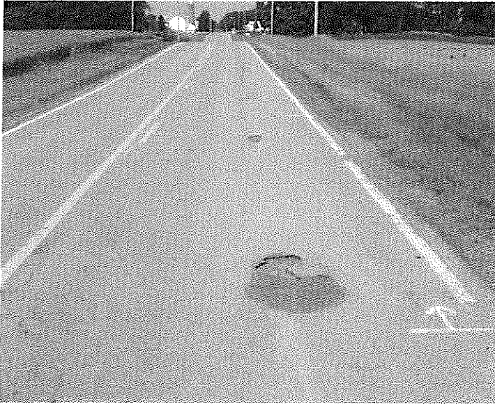
Looking East on Kramer Rd. There is a hole in the pavement.
