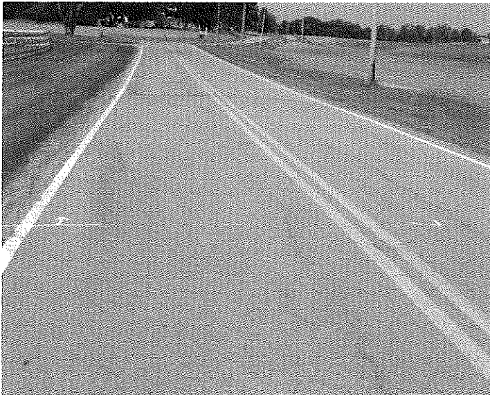
Looking West on Kramer Rd. The pavement is cracking and there is wheel rutting across the road.
