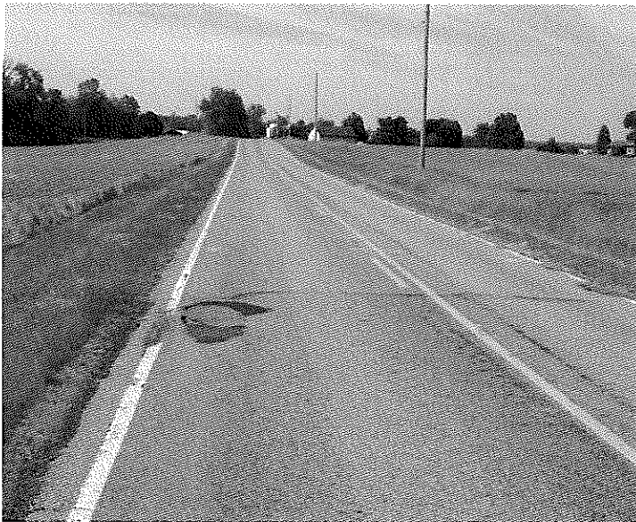
Looking West on Conkle Rd. There is wheel rutting across the road.
