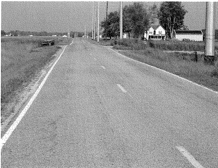
Looking West on Ft St Road. There is wheel rutting across the road.
