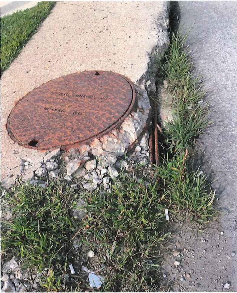
One of the existing No. 2-6-A inlet upper boxes that needs replaced.
