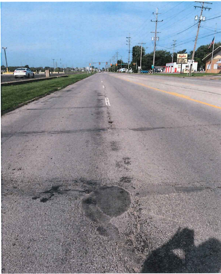
Oxidized pavement with longitudinal and transverse cracking. Repaired potholes.
