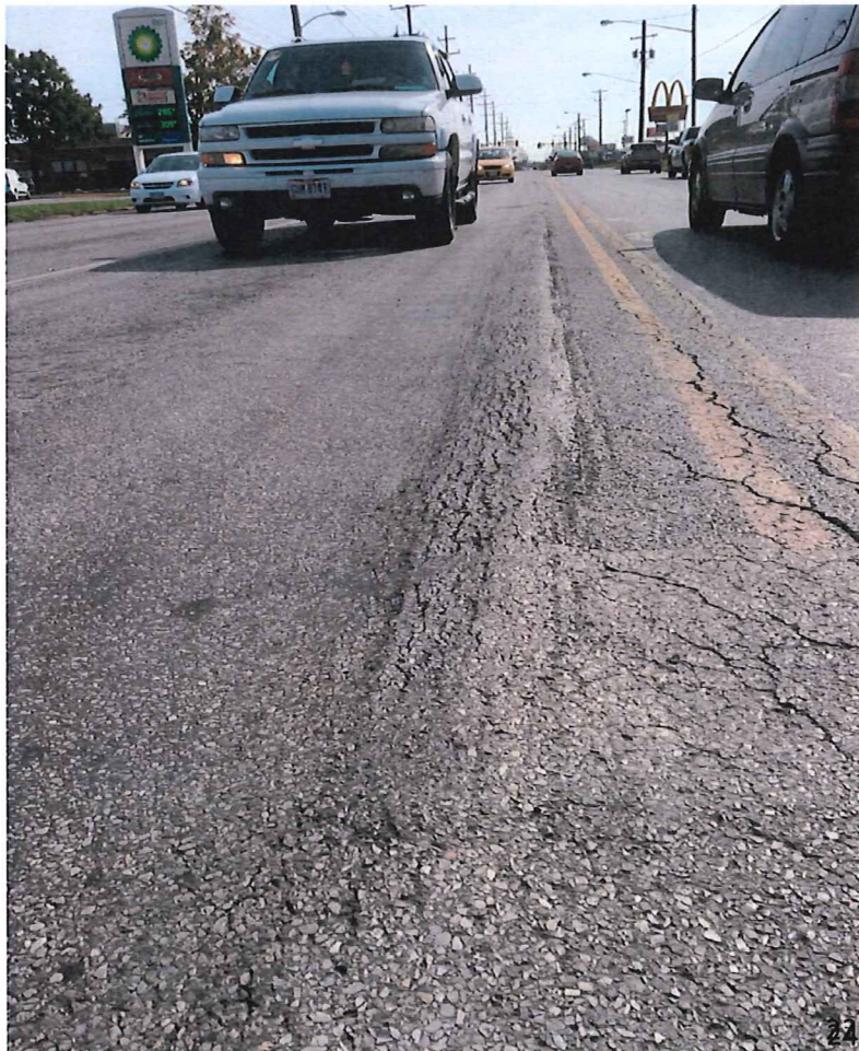
Moderate rutting at the westbound left turn lane on Perkins Avenue at SR 4.
