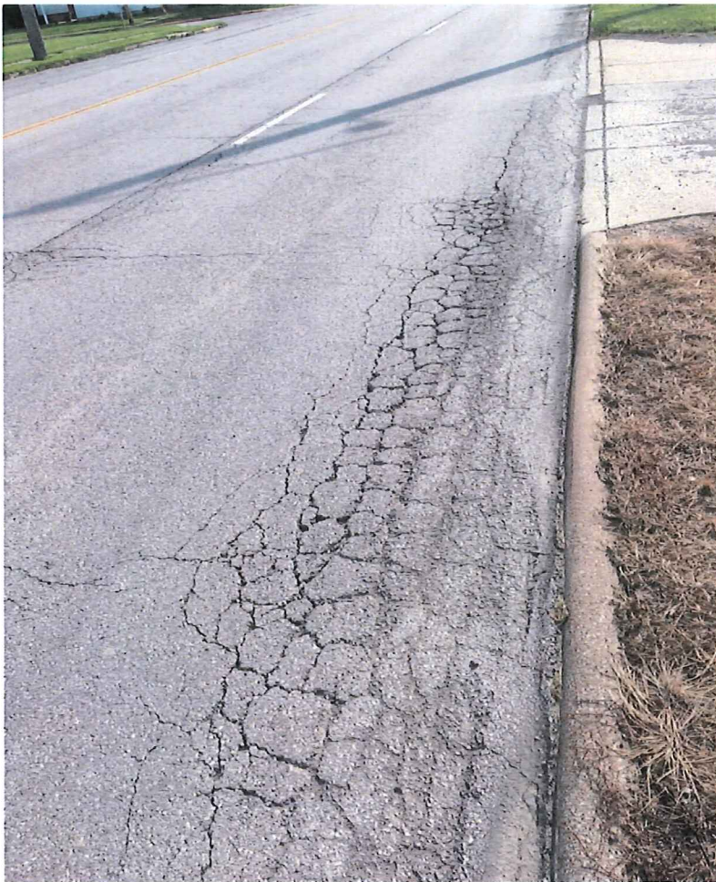
One of the many areas exhibiting alligator cracking.
