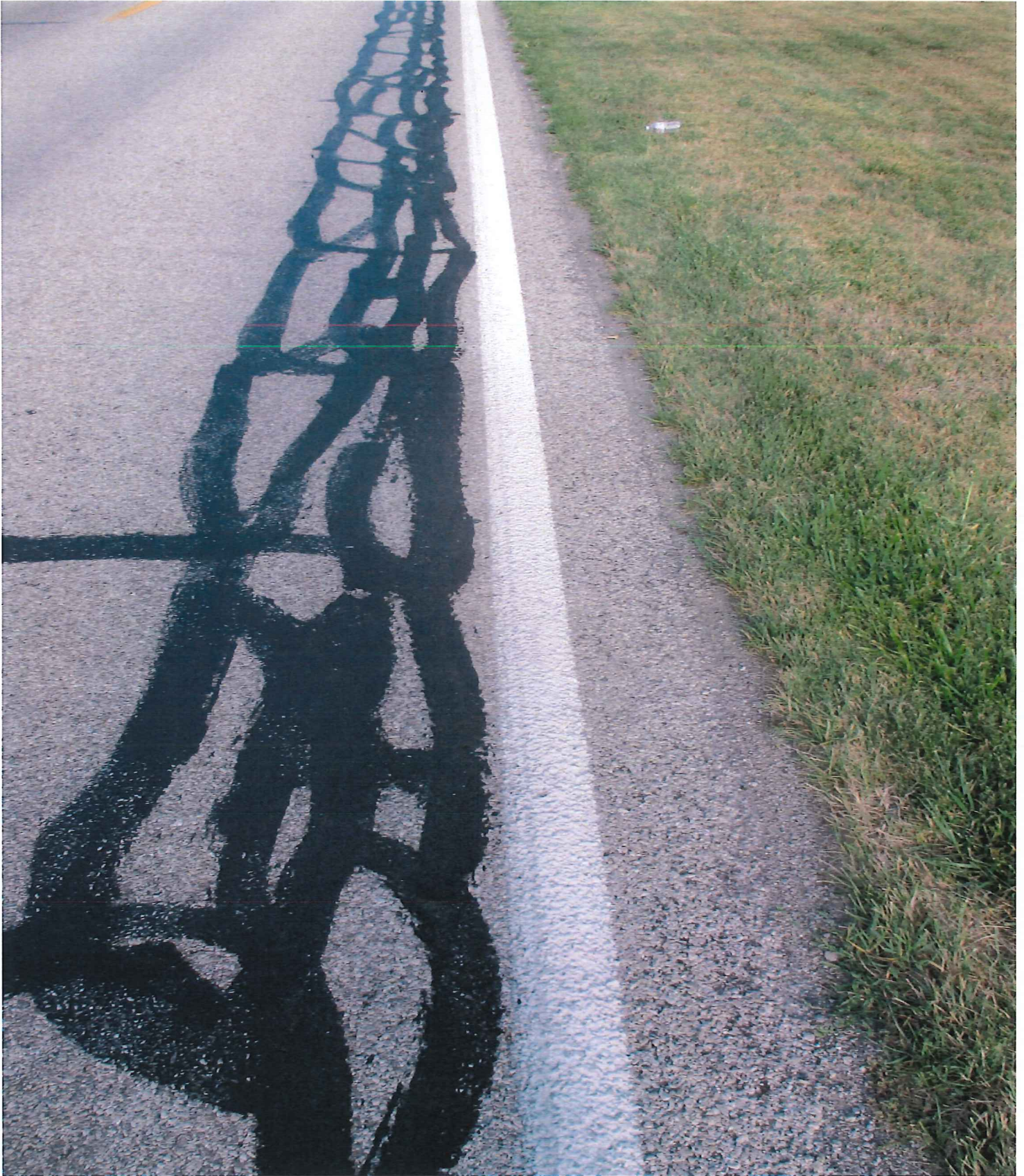
Heavy wheel path cracking.
