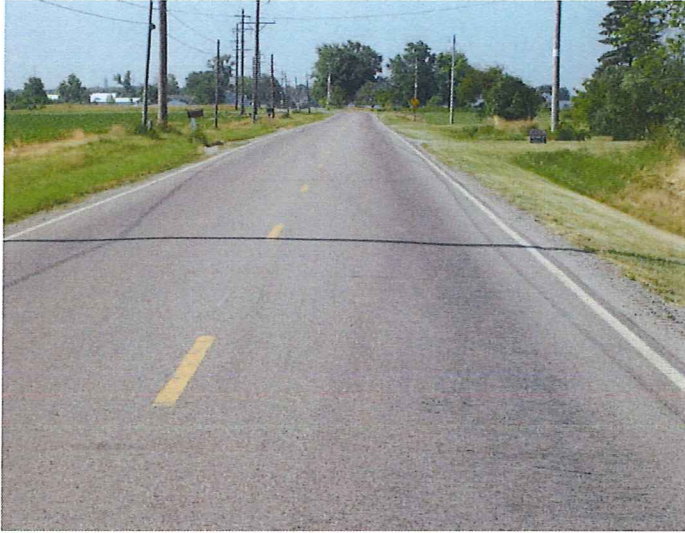
Looking South on Hicksville Edgerton Rd. There is wheel rutting across the road.
