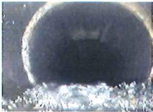
Offset pipe joint leaking
