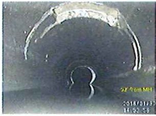
Defect in pipe
