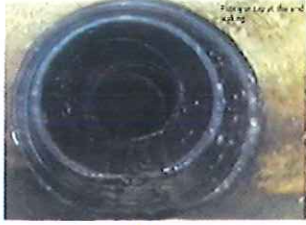
Cap or fittings leaking
