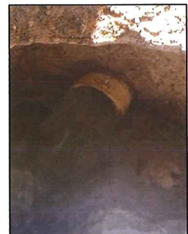
Figure 5. 4-inch invert flowing full into manhole
