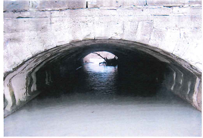
Columbus Ave. Structure P-209. Deterioration of block joints and mortar loss. Pneumatically applied concrete placed on some faces in the 1980s in an effort to slow joint deterioration.
