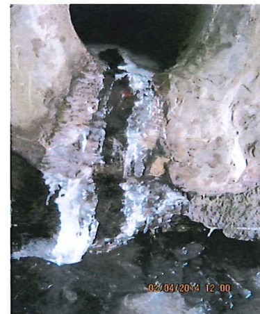
Columbus Ave. Structure P-209. Deterioration of stone at storm sewer outlet on interior of arch span.
