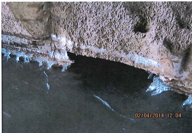
Columbus Ave. Structure P-209. Deterioration of stone blocks on structure interior.
