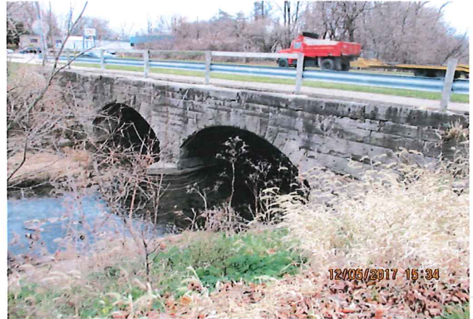
Columbus Ave. Structure P-209. General view of bridge. Bridge is a two-span filled spandrel masonry arch (total span 40').
