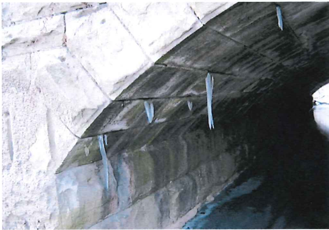
Columbus Ave. Structure P-209. Leakage through stone block joints leading to deterioration and loss of mortar.
