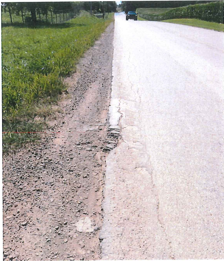
Edge and longitudinal cracking the entire length of the pavement.
