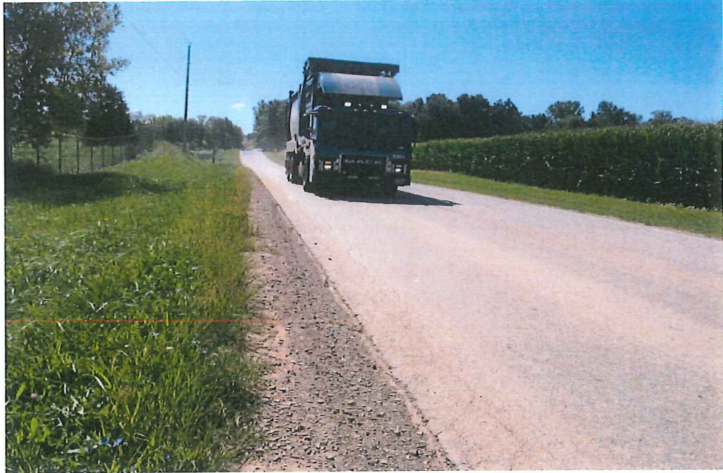
Edge and longitudinal cracking the entire length of the pavement. Hoover Road is the road leading to the Erie County Landfill.
