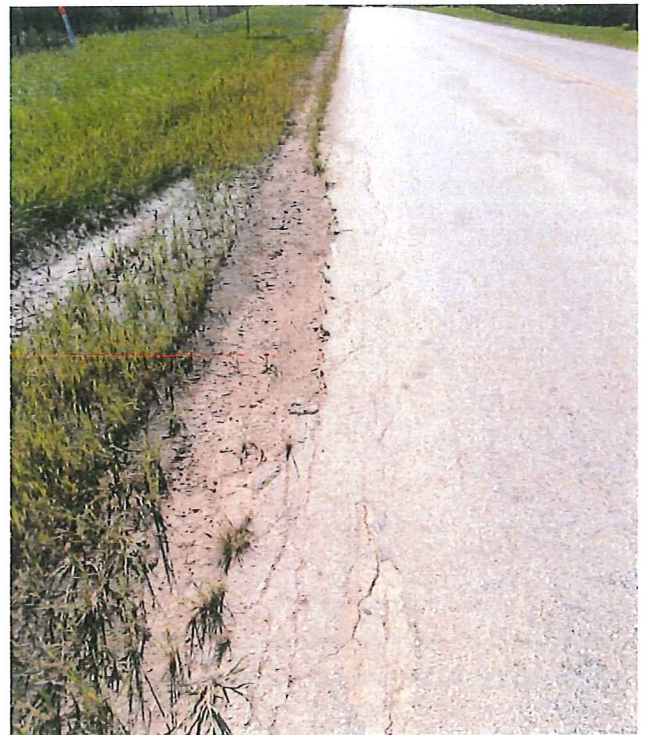
Edge cracking resulting in missing asphalt.
