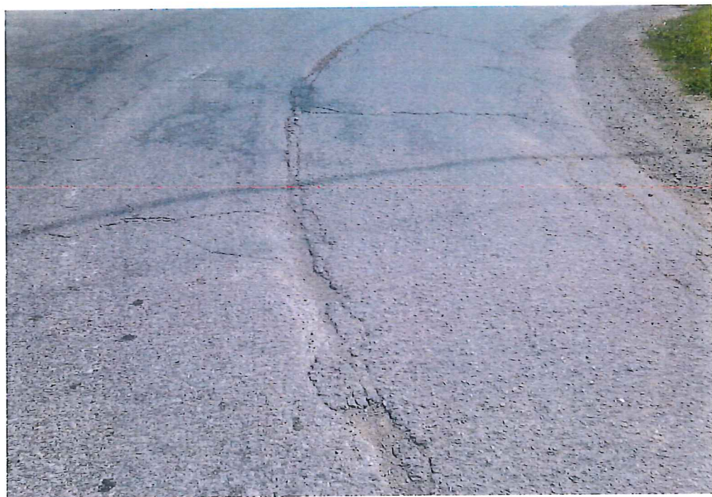
Pavement cracking on Hoover Road at the Huron Avery Road intersection. This is the primary route to the Erie County Landfill for garbage trucks.
