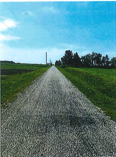
Road 5A - Various locations of cracks and patches
