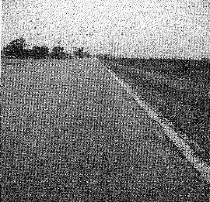
Looking North on Harris Rd. There is wheel rutting.
