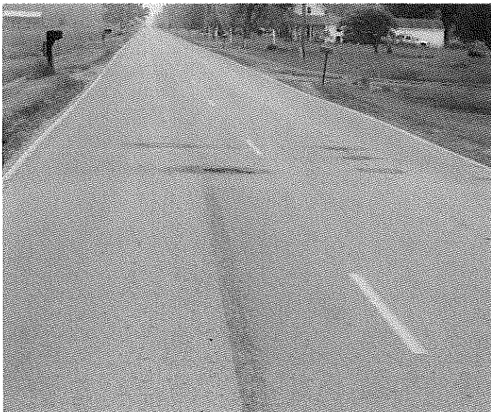
Looking South on Harris rd. There is wheel rutting across the road and holes in the pavement have been filled.
