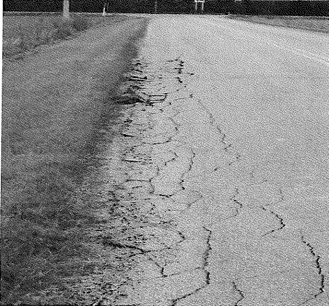
Looking North on Schubert Rd. The edge of pavement is cracked.
