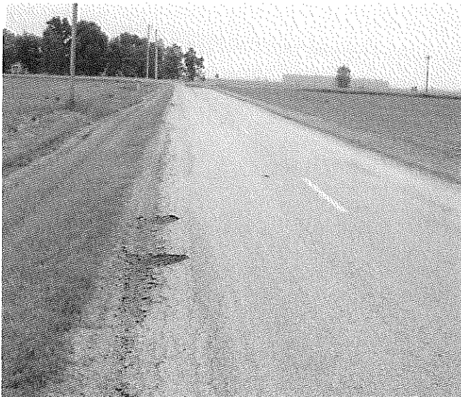
Looking north on Harris Road. The edge of pavement is cracking and there is wheel rutting across the road.
