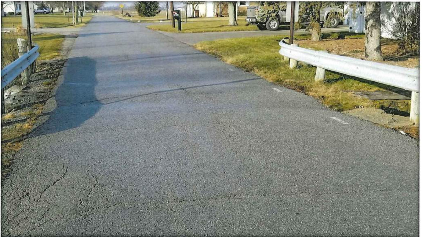
PAVEMENT SEETTLING ON BOTH SIDES OF CULVERT
