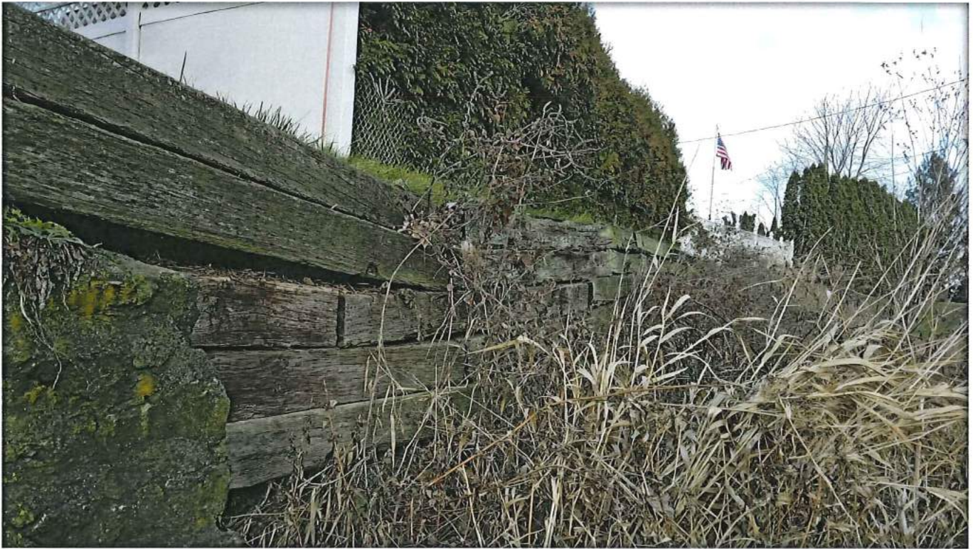
TIMBER RETAINING WALL IN NW CORNER IS SETTLING WITH FILL MATERIAL WASHING THROUGH
