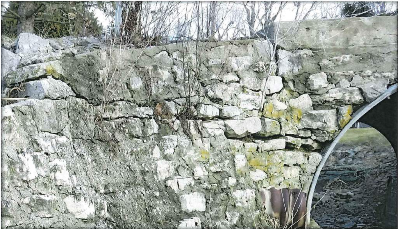
LOSS OF MORTAR BETWEEN MASONRY STONES SW WING WALL
