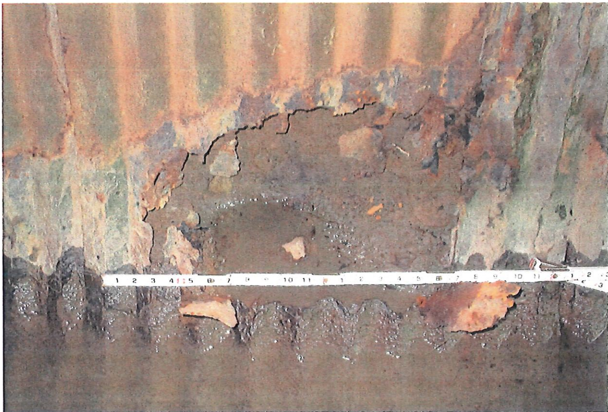
Large areas of complete section loss in multiple locations in pipe allowing backfill to infiltrate in from behind culvert. Backfill material missing from behind pipe in areas of large holes.
