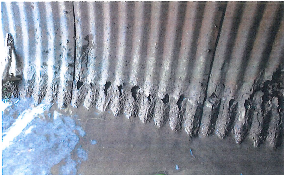
Extensive heavy rust and scaling throughout pipe bottom. Holes and perforations thought out on both sides along flow line around 25% of the total area. Large holes in multiple locations on South side of pipe.
