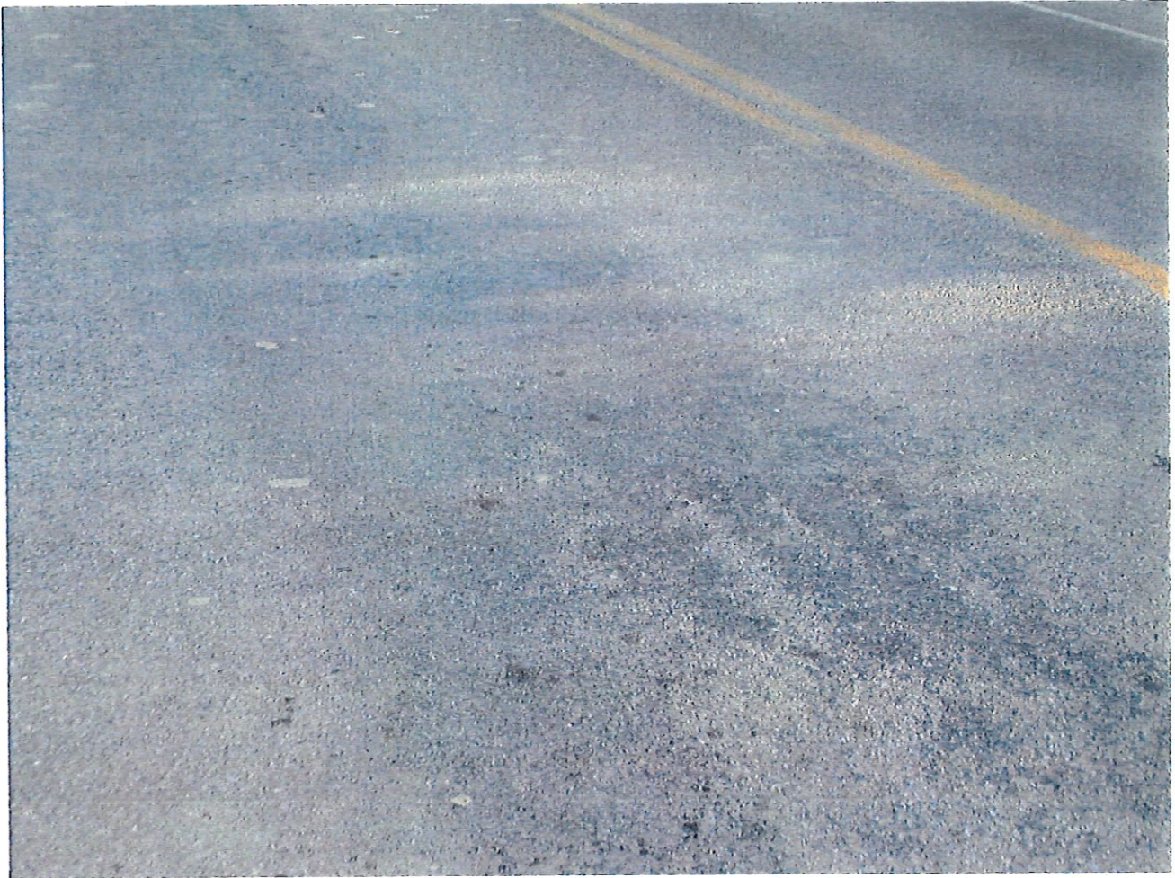
Oxidized and raveling pavement showing distresses in pavement surface course.
