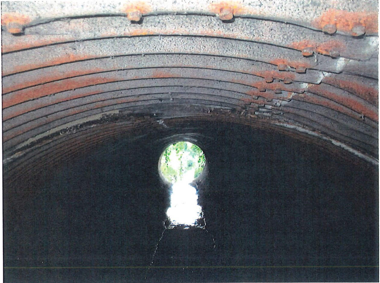
Slight shape deflection in top of corrugated metal culvert with heavy rust.
