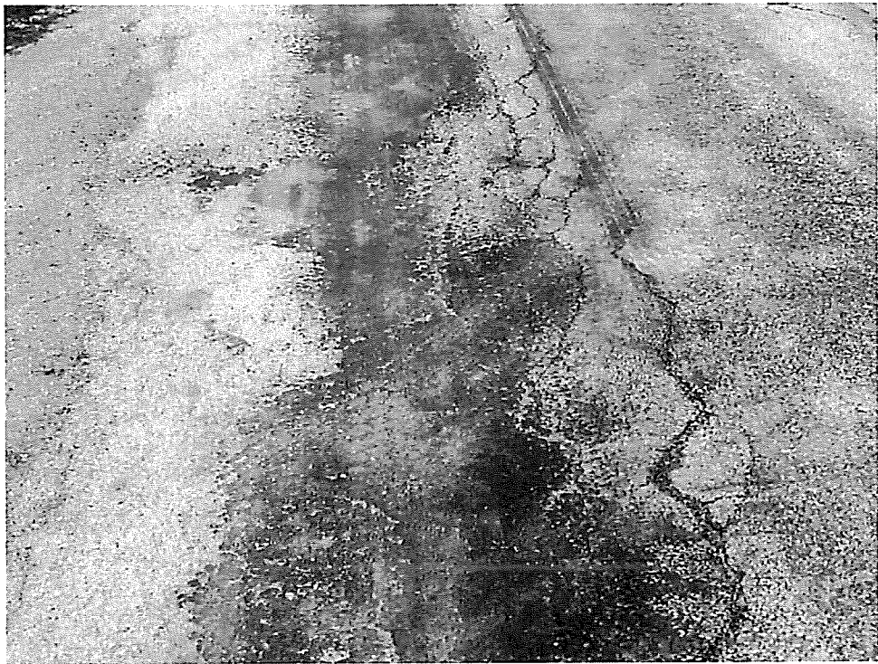
Photo 2 – Failed Edge Repairs
