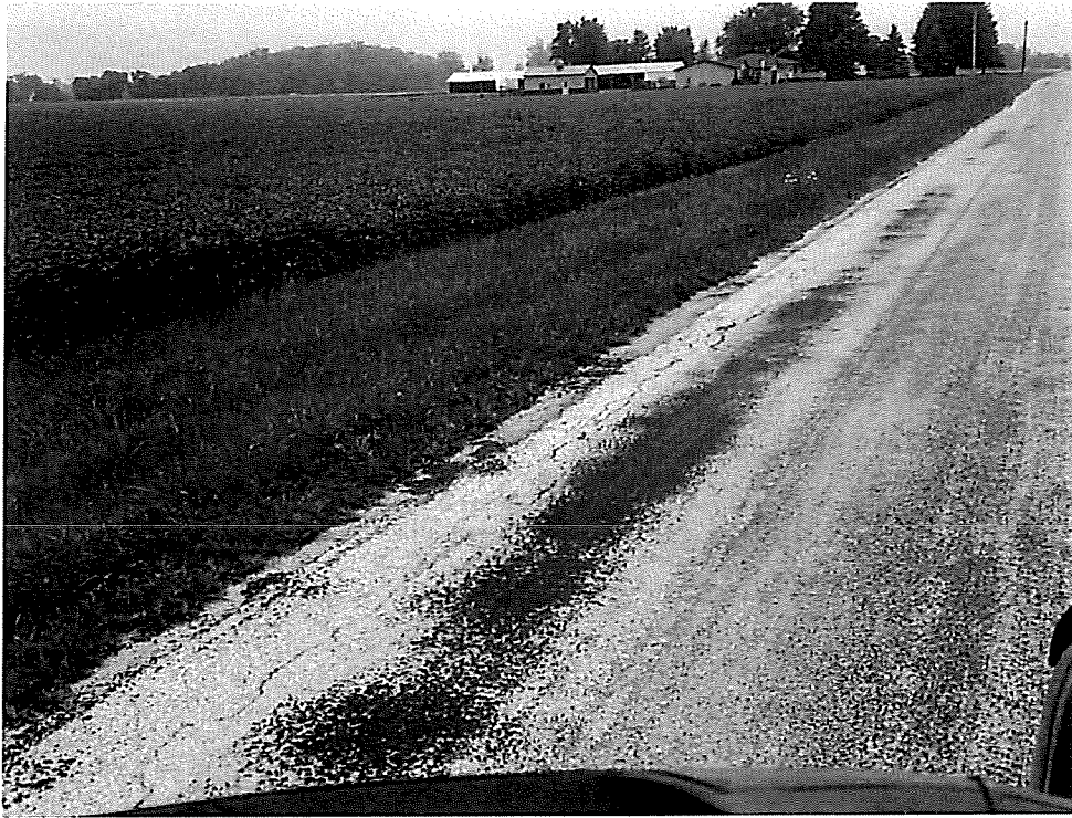
Photo 1 – Edge Failures with Bleeding
