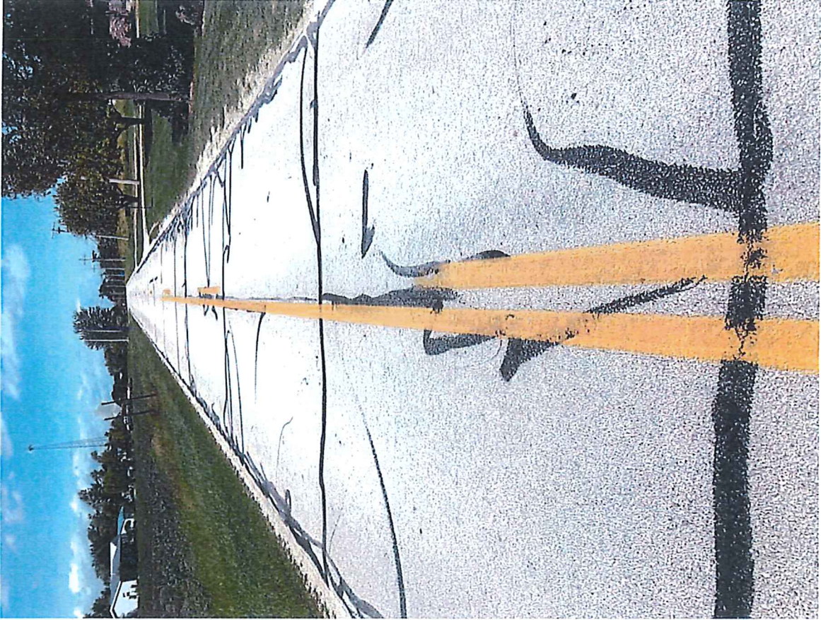
Photo 5 – Widespread Transverse, Edge & Random Cracking
