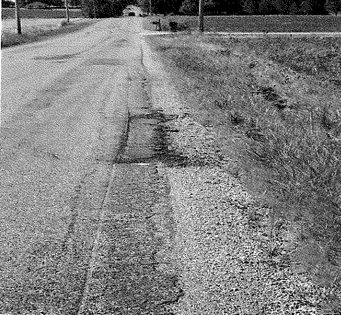
Looking south on Ridenour Road. The pavement is cracking and chipped.
