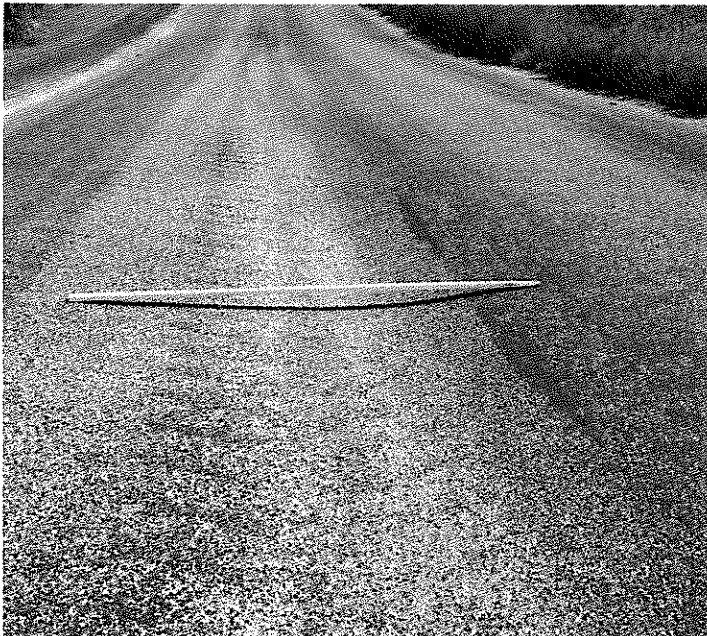
Looking north on Ridenour Road. There is wheel rutting across the road.
